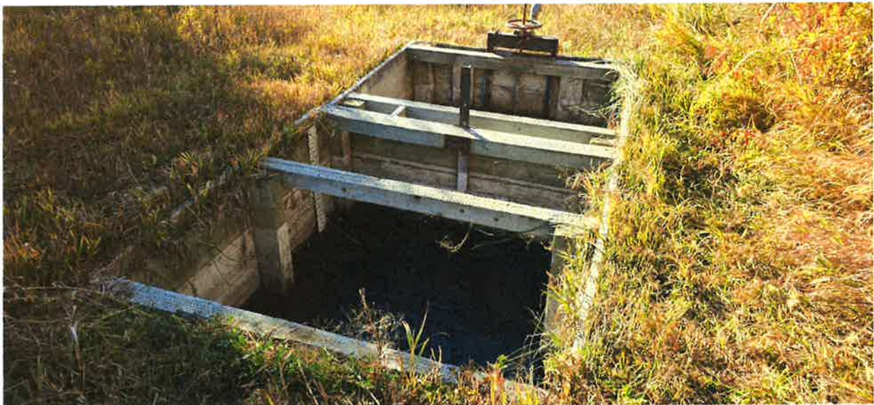
Figure 2: Measuring device and Headgate (downstream side)
