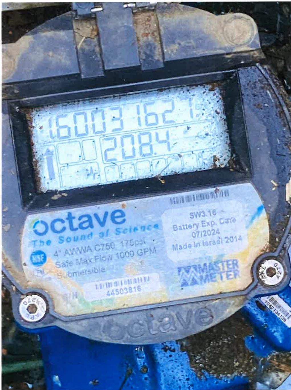
Installed flowmeter showing flow rate at time of exam (208.4 gpm, or 0.46 cfs)
