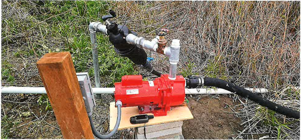
Figure 2: 2 Hp pump and filter adjacent to Snake River
