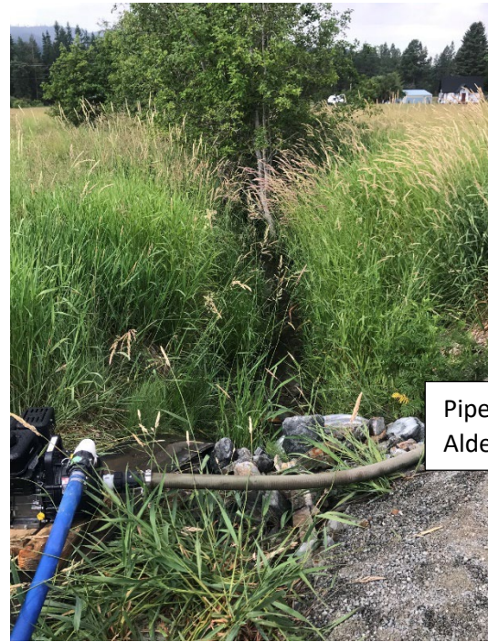
Pump from Alder Creek looking downstream
