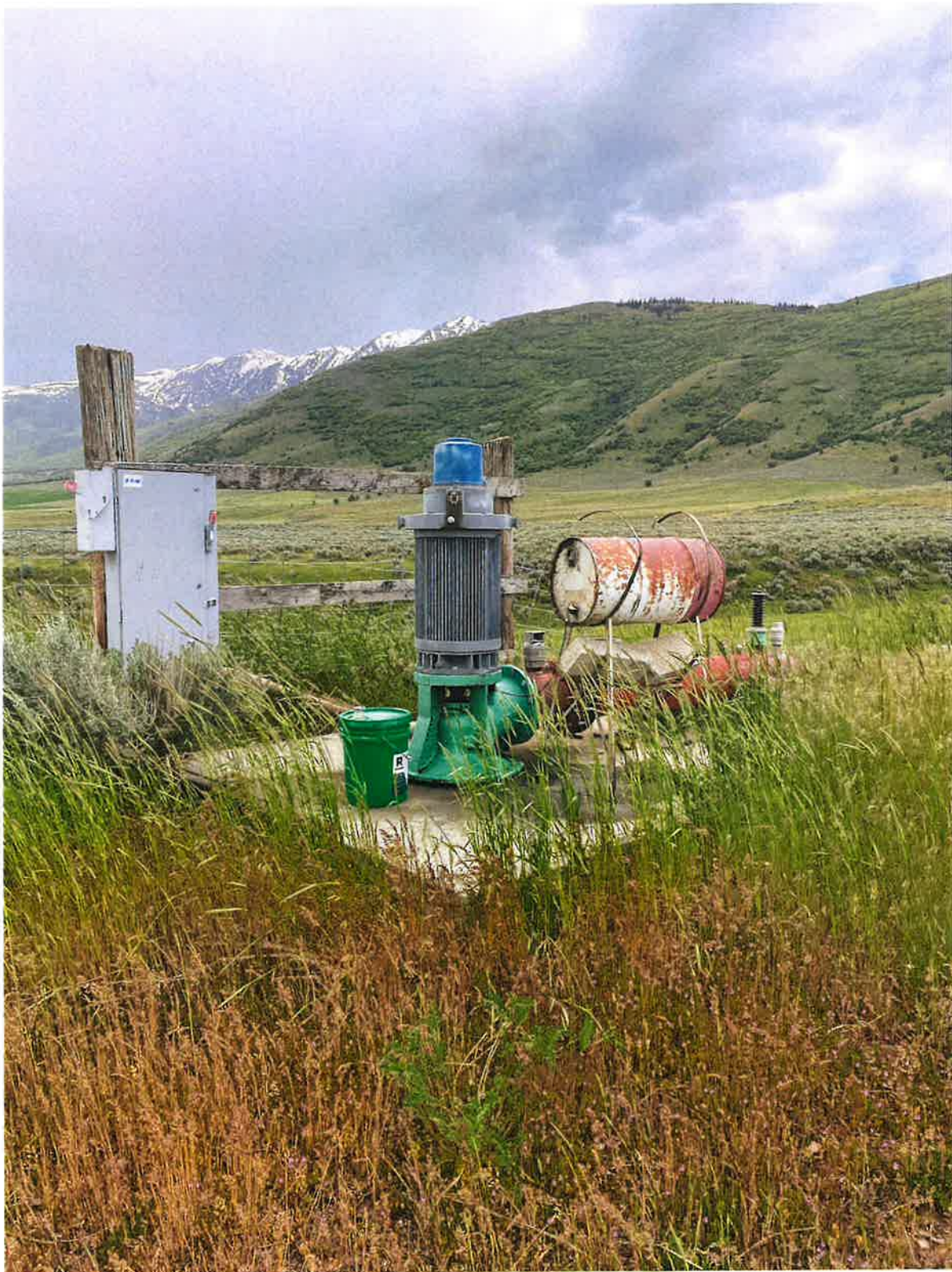
Irrigation Well SW of House – Well 1
