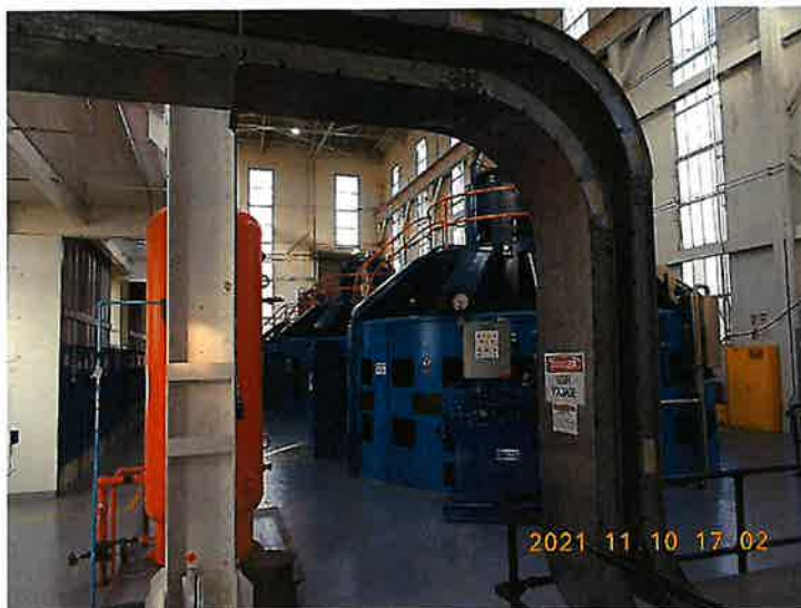
Photo 1. Three turbine/generator units currently in place.
