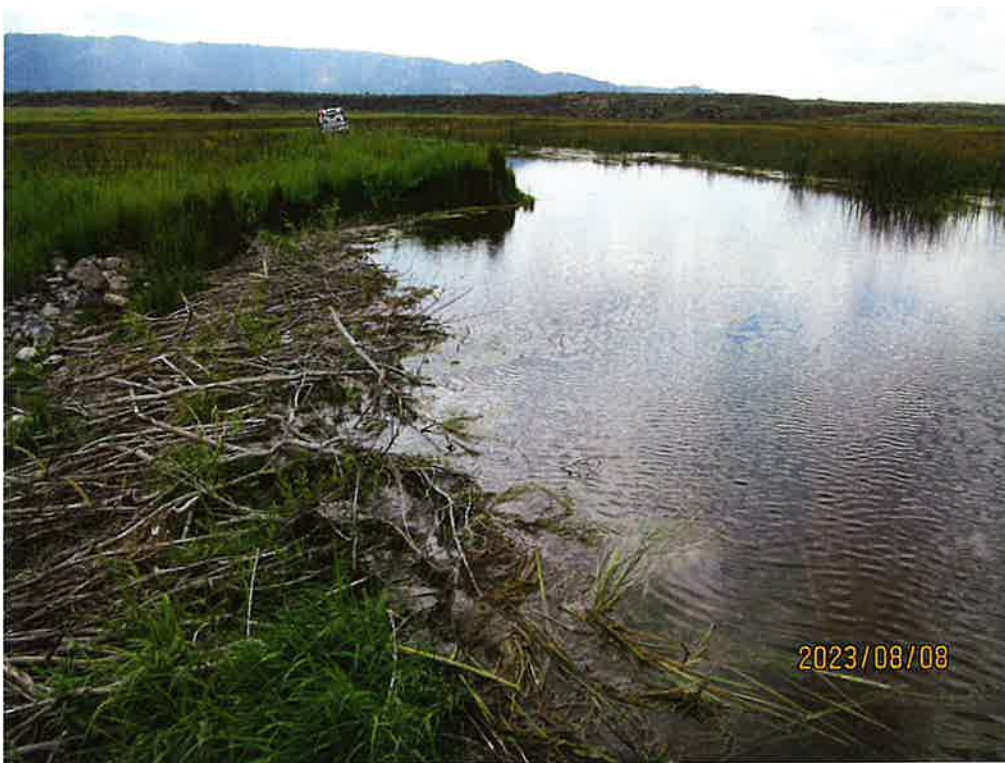
Photo 2. Looking West at north berm. Beaver activity heavily built over gabion structure. Water flows over structure.
