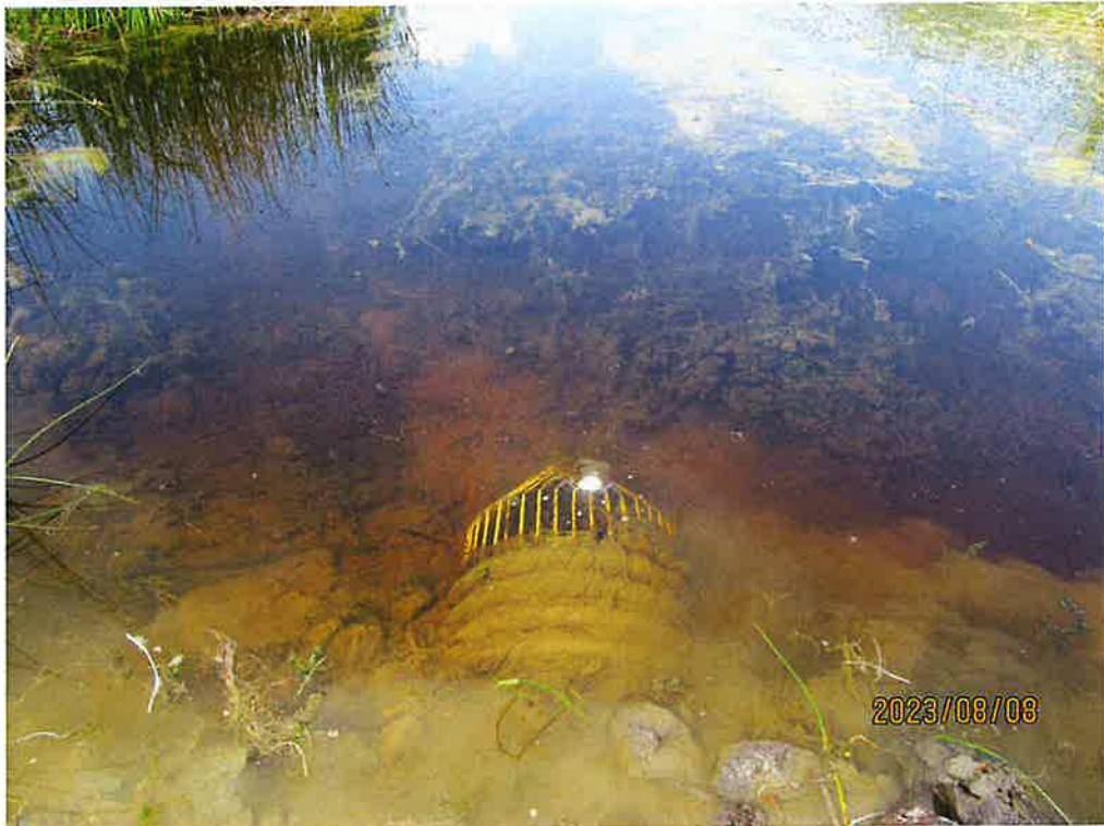
Photo 5. Submerged inlet structure of large reservoir, looking upstream.
