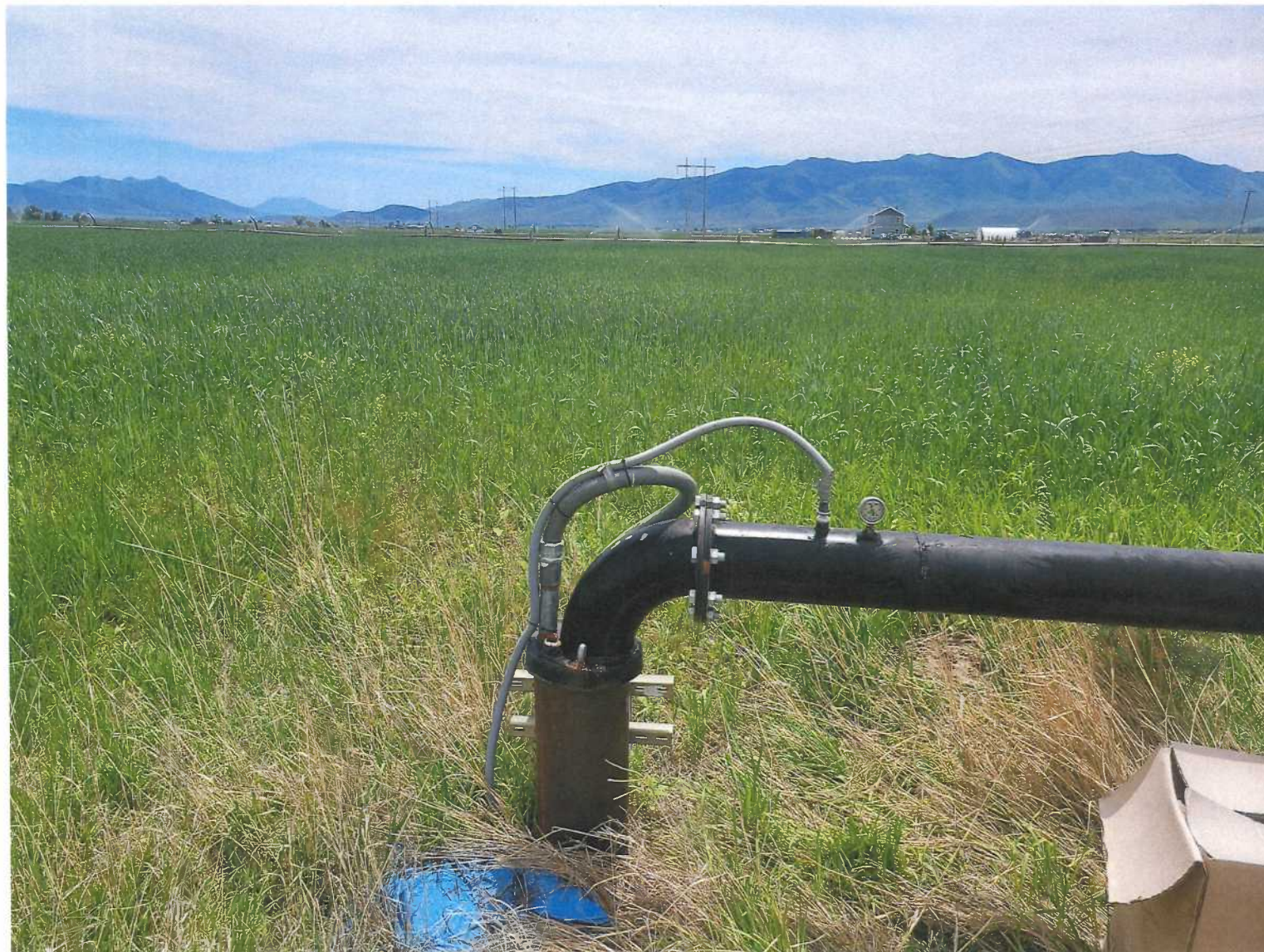
30 HP Submersed Pump in [NW]SESE Wheel lines in background Metal Tag No. D0074184
