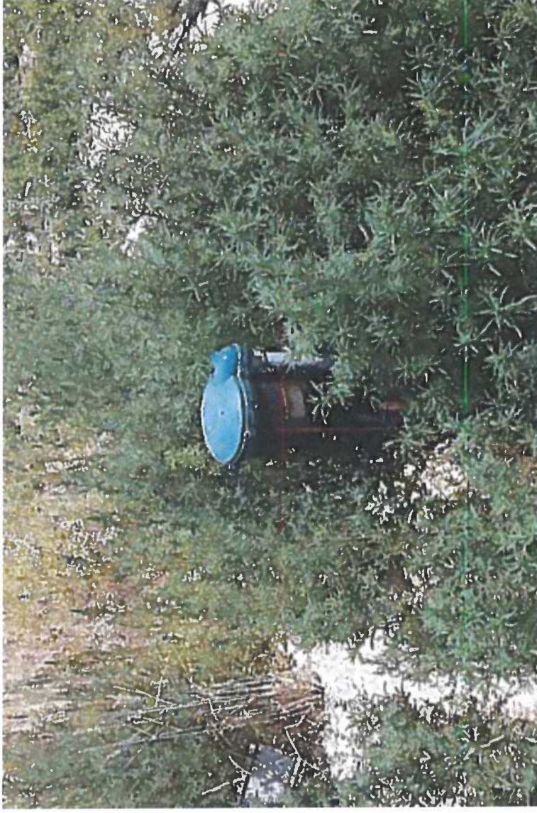
15 HP Submersible Pump in [SW]SESE Tag No. D0068300
