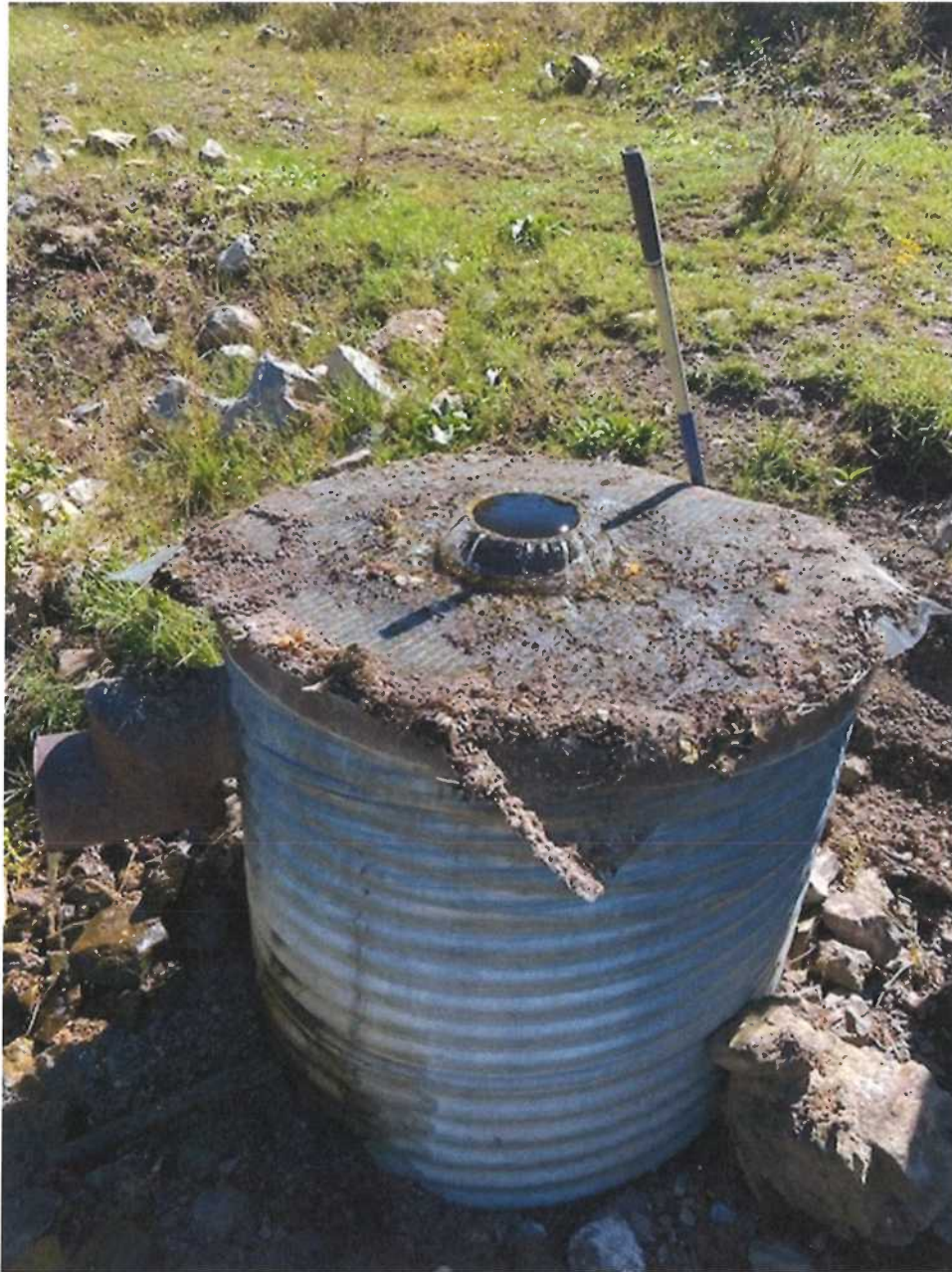
Vertical storage tank, debris filter, beginning of small pipeline and main pipeline
