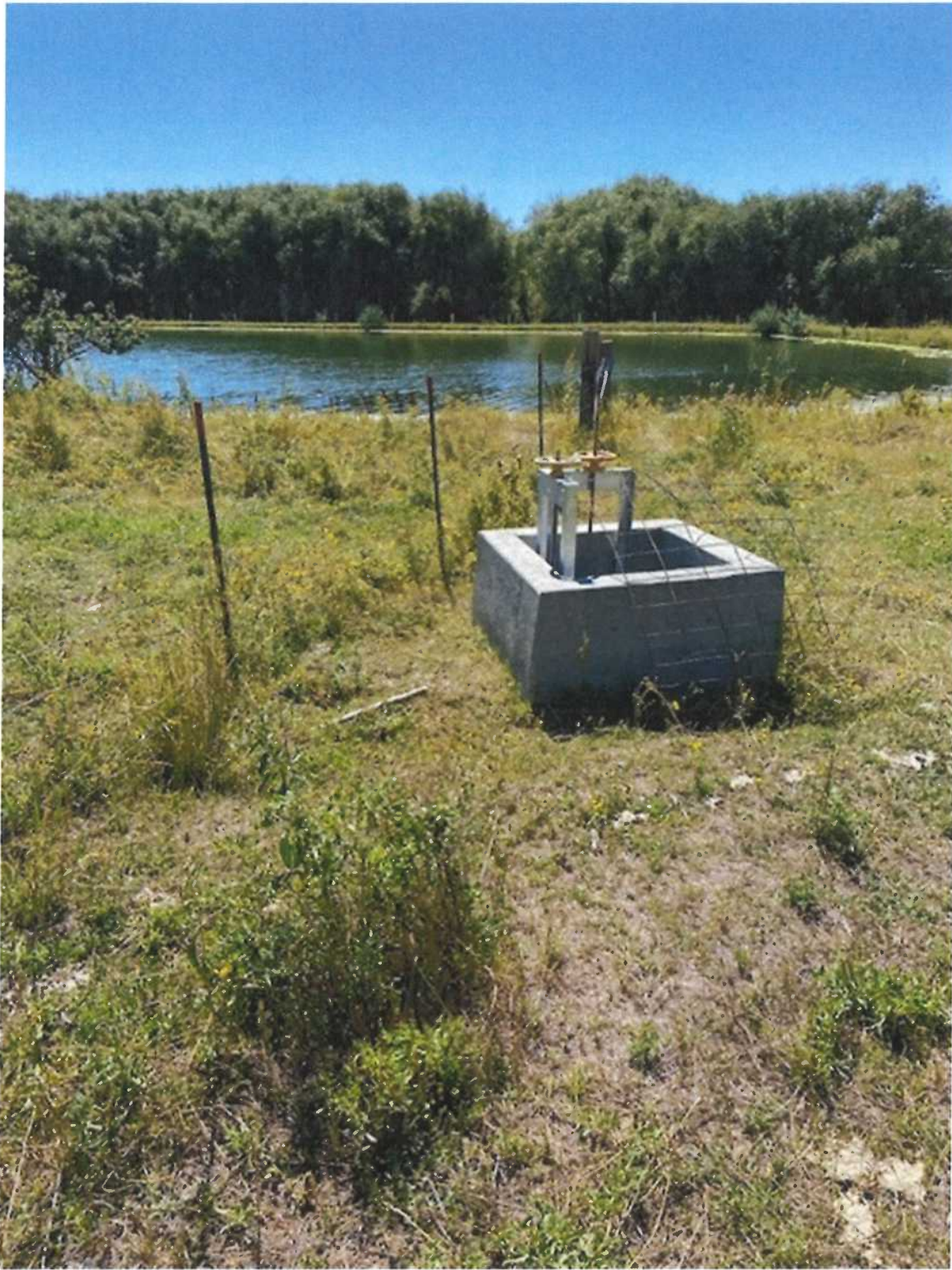
Control box on buried pipeline.
