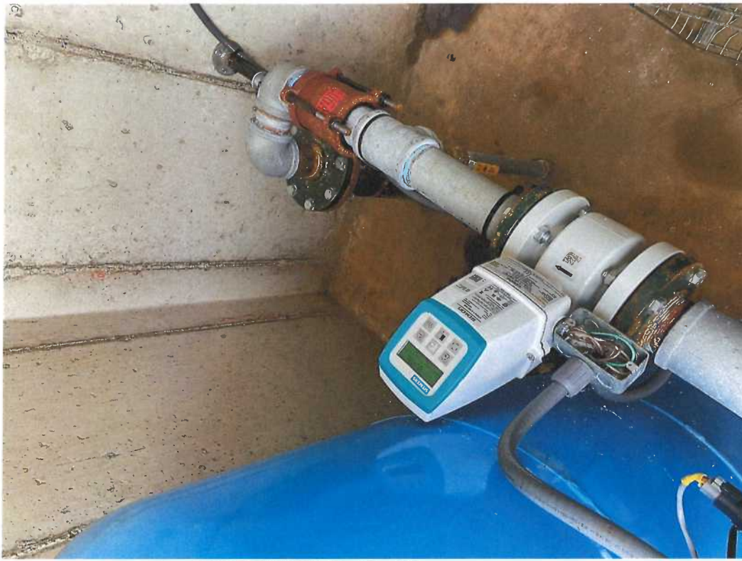
Flow meter installed on large well in concrete vault.
