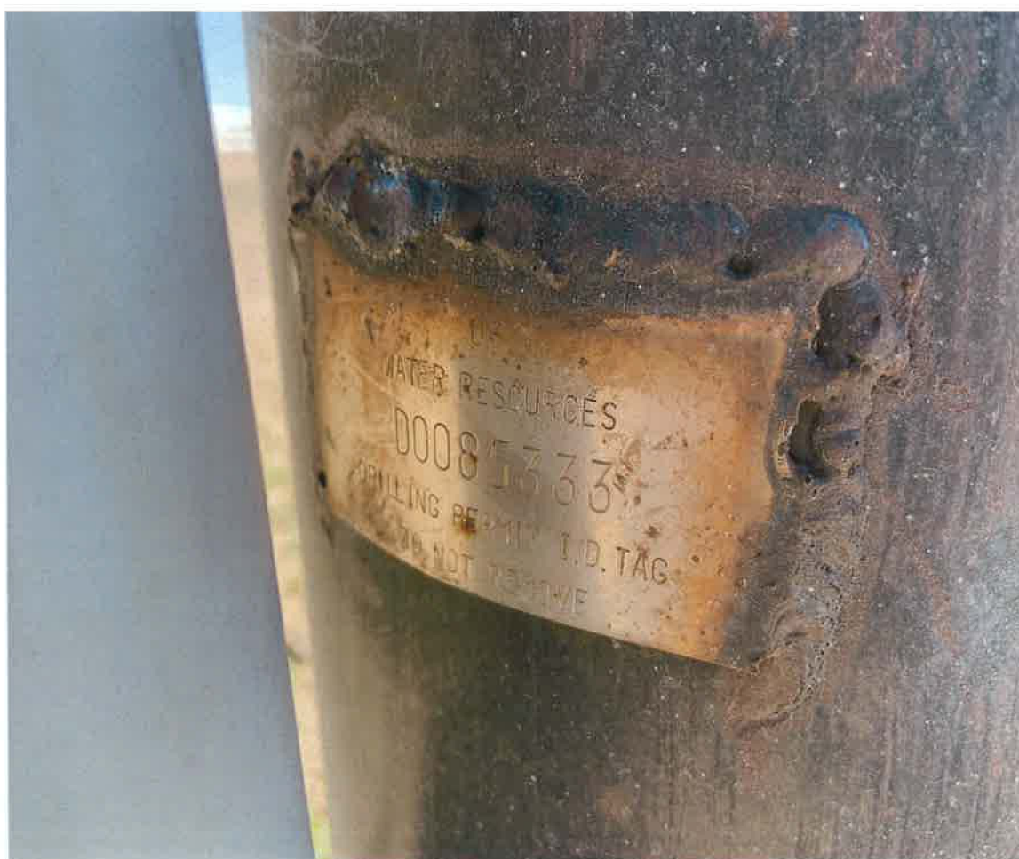
Fig. 4 - Well Tag ID D0085333 43° 10' 5" N 115° 43' 23" W 60 HP submersible pump
