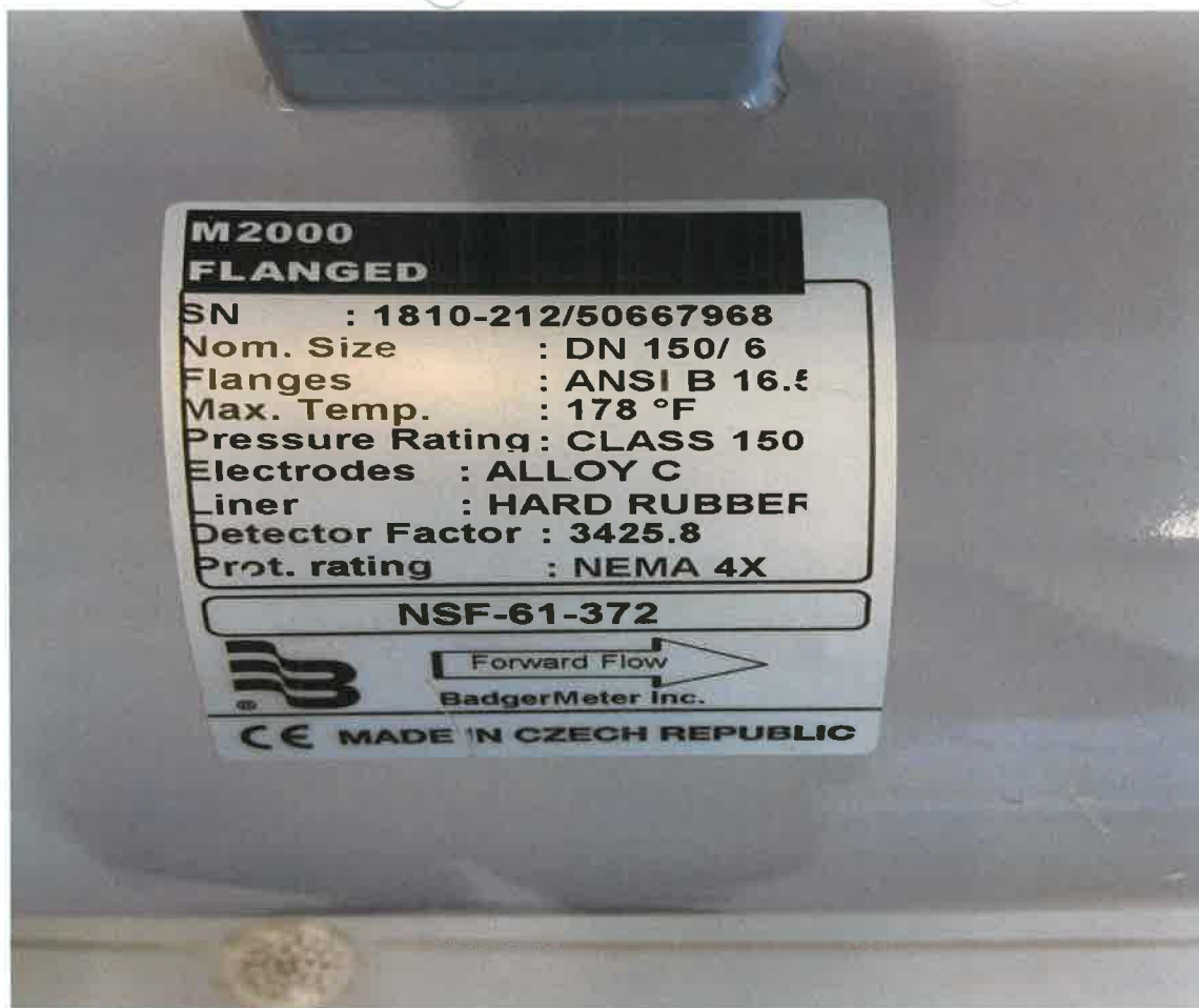
Fig. 5 – Specs for measuring device installed on central line from both wells.
