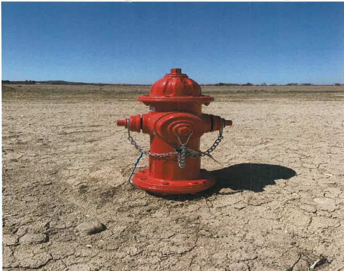
Fig. 11 – Nine standard fire hydrants are installed throughout the subdivision for fire protection. Hydrants are spaced approx. 500 ft. apart.
