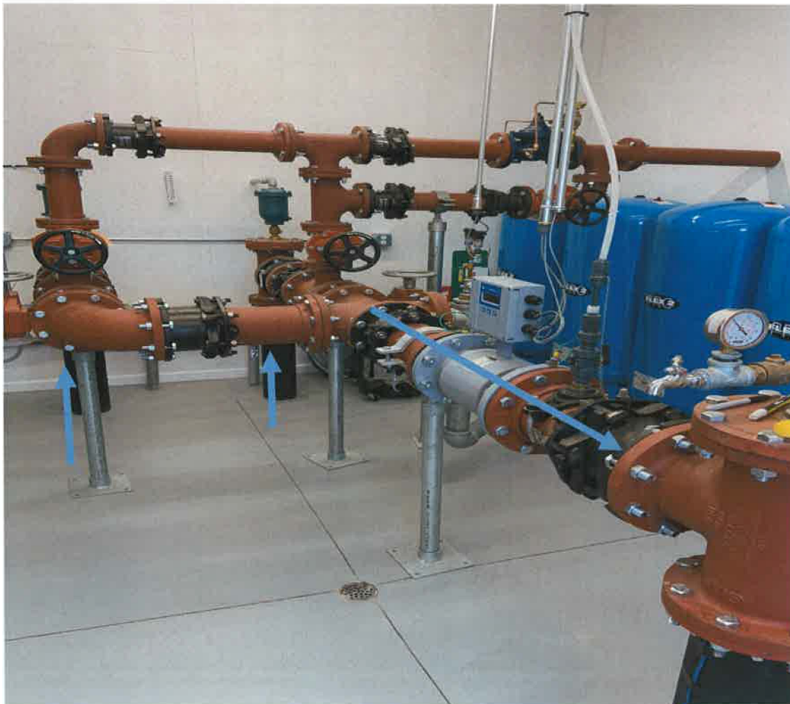
Fig. 8 – View inside of pump house. Water comes in from the two wells in the background and into the pressure tanks. Water then goes from pressure tanks to single line with flow meter out to delivery system under the streets of the subdivision.
