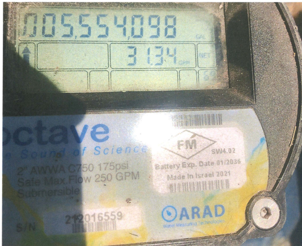
Figure 4 Pump setting allows for 31.34 GPM. Photo provided by water user.
