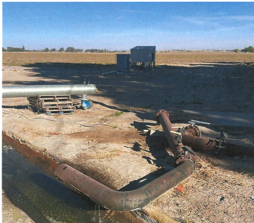
Figure 7 Diversion system including well house (point of diversion) and the open-ended pipe that delivers water to the ditch from well. Photo taken facing North.
