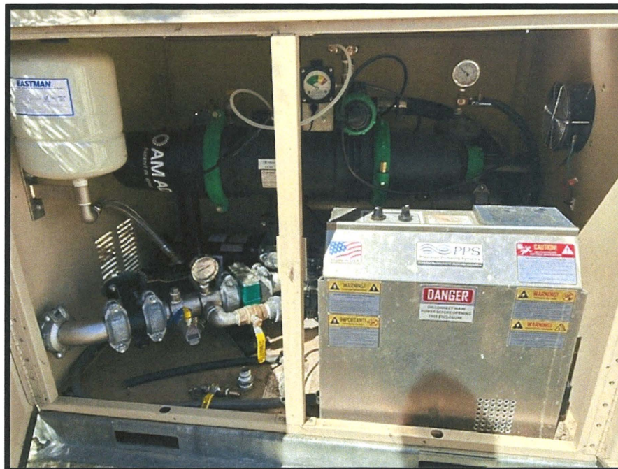
Figure 5 -Irrigation Photo C of the pump with VFD controller submitted by the permit holder.
