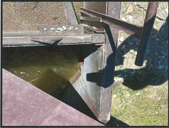
Photo 5- At the center of the image the overflow orifice visible below the fish screen enclosure. The orifice slip panel handle is seen installed on the right side of the screen enclosure.
