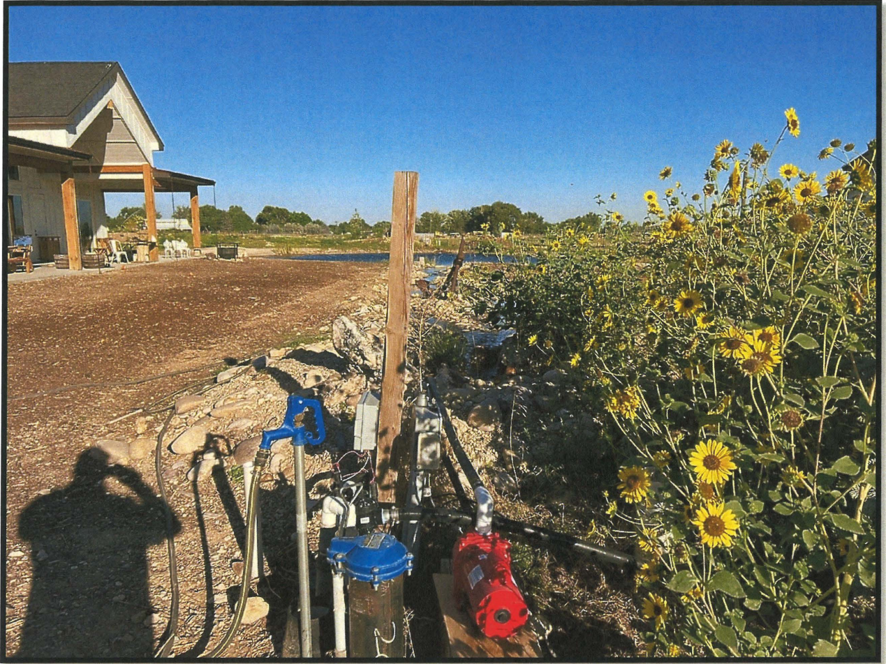
Photo 10- c.2024- Taken at the well head facing west towards the pond. Red recirculation pump is visible to the right of the well head. The white PVC manifold on the left of the pump has 2" poly lines with valves feeding the lined ditch that empties into the pond, the 11 wind fighter sprinklers on risers just north of the ditch, and the driplines for the orchard in the southeast corner of the parcel. A separate buried line supplies the home and sprinklers directly to the south of the home.
