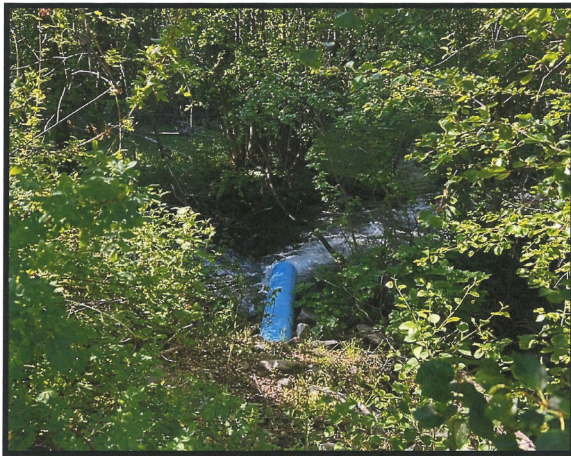
Photo 5- 10" PVC fish bypass pipe returning flow to Pratt creek about 20 ft east of the fish screen enclosure.
