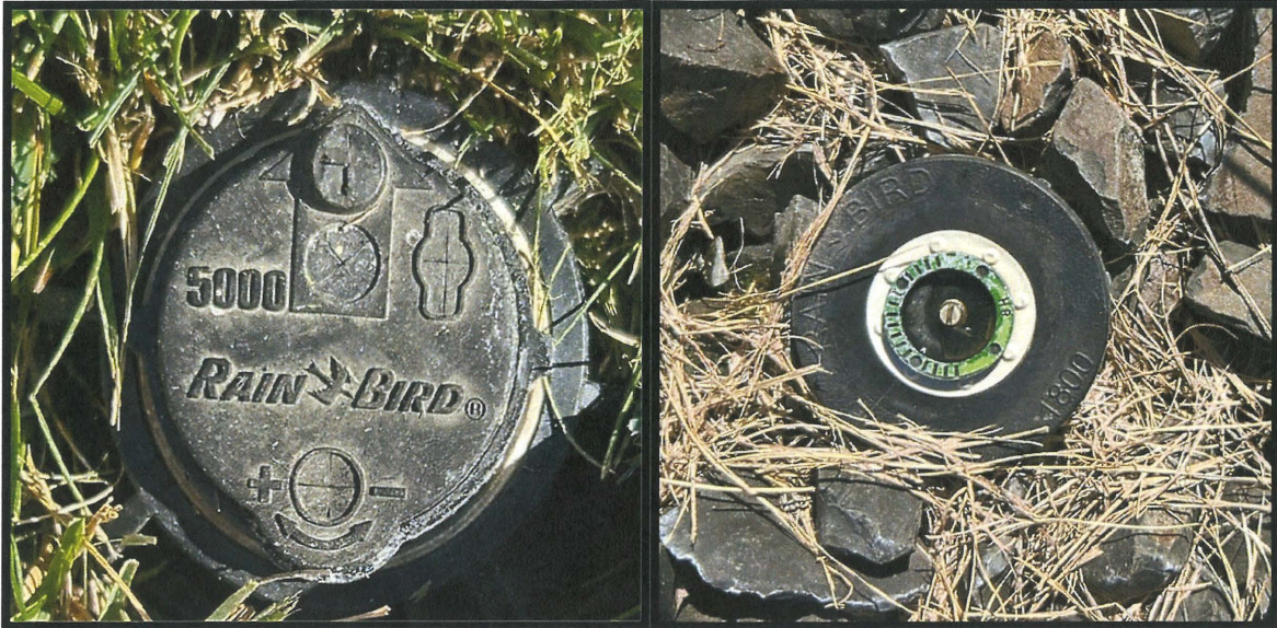
Photo 4 (Left) - Rain Bird 5000 series rotary sprinkler heads found throughout the larger zones in the POU. Photo 5 (Right) - Smaller Rainbird 1800 umbrella sprinkler head like those found in the landscaped beds of the POU.
