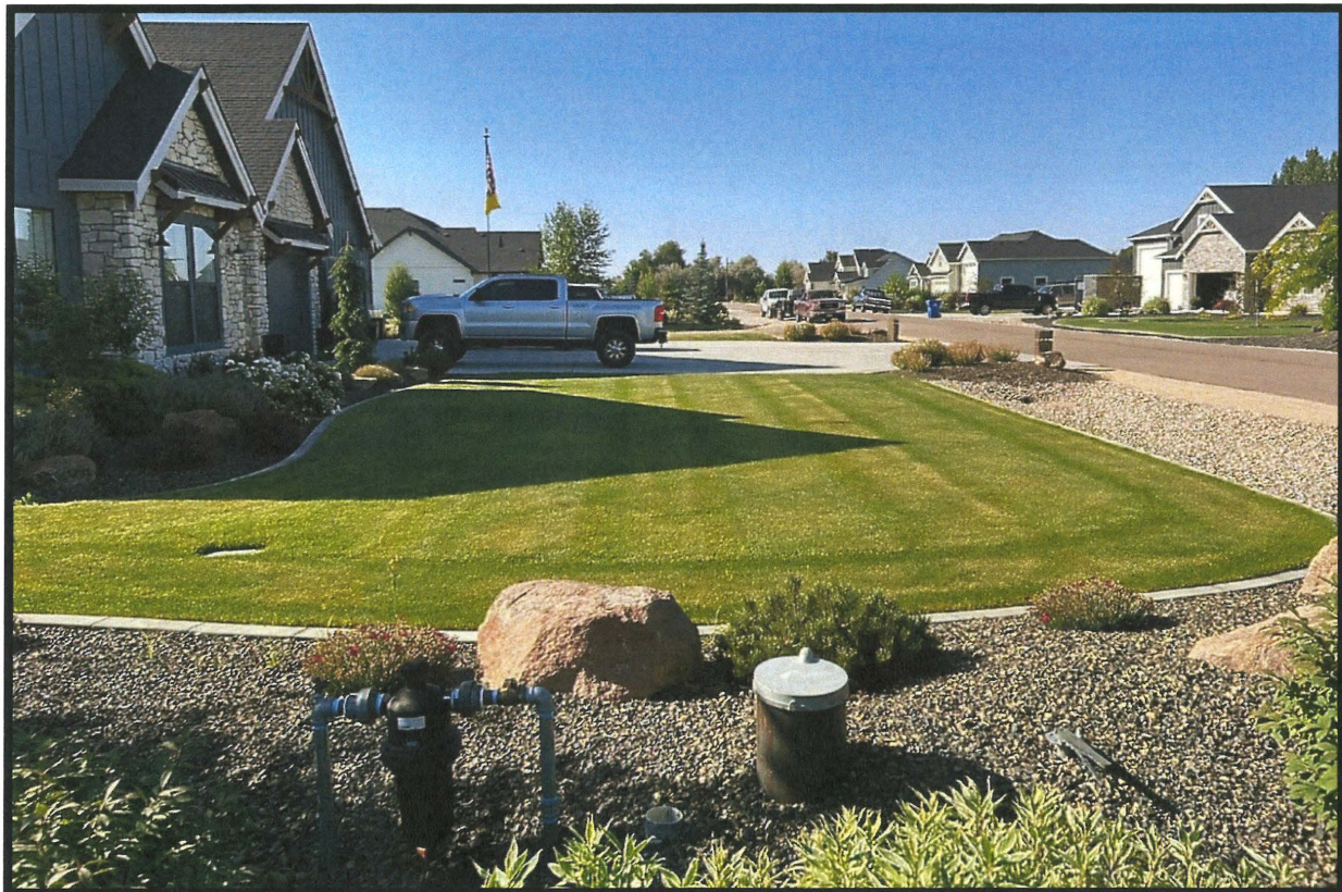
Photo 1 -Shallow well head with butterfly shutoff valve on the left in image. The 1 1/4" irrigation line with a bowl filter conveying water for the sprinkler system is left of the well head. Taken Facing south at the northwest corner of the parcel.
