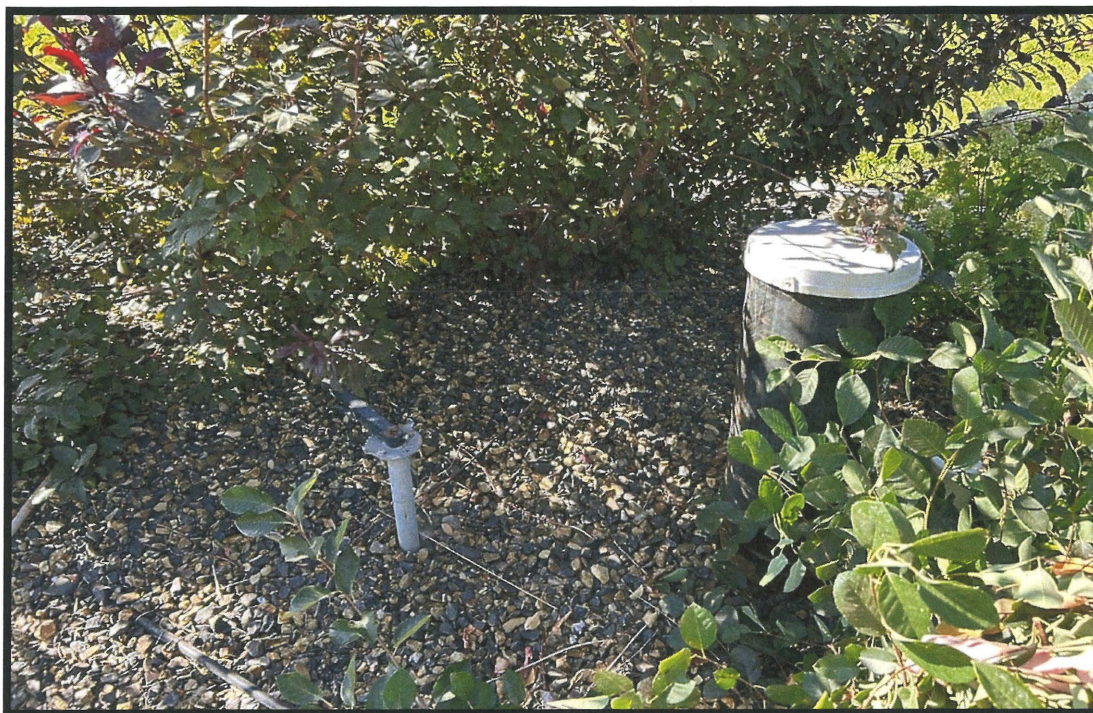
Photo 1 -Shallow well head with butterfly shutoff valve on the left in image. Taken Facing south at the northeast corner of the parcel.
