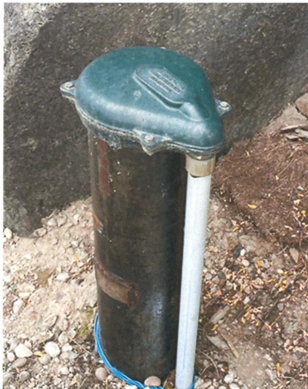
Figure 4 Well head that serves as the point of diversion for this license.
