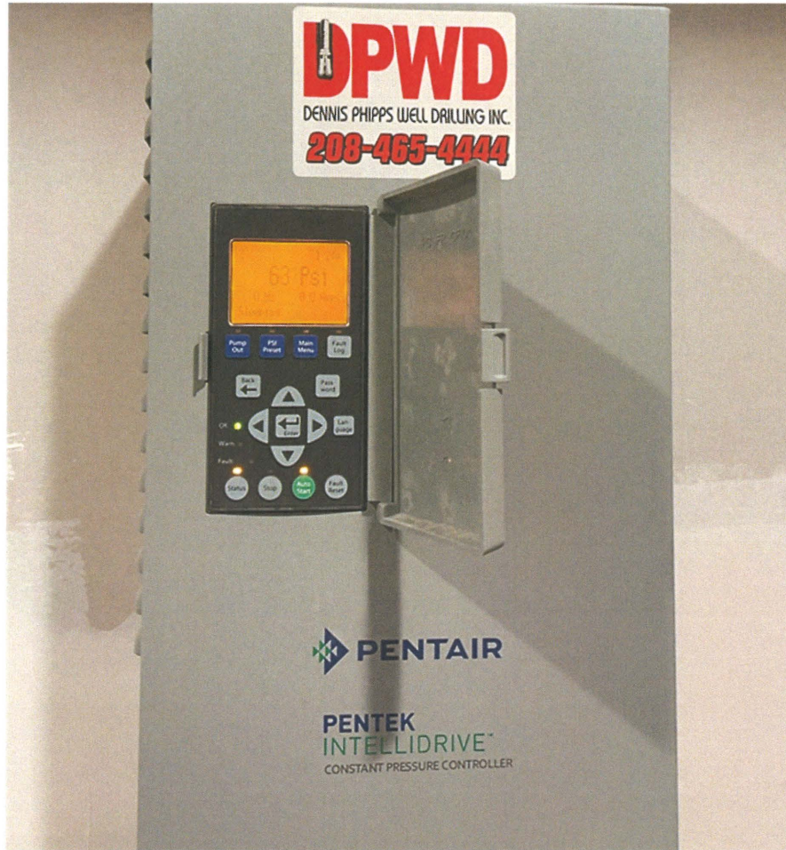
Figure 7 Front view of well pump motor control box showing system setting at 63 psi.
