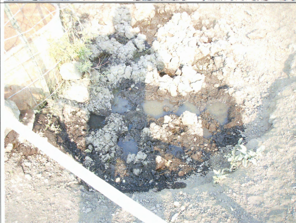
Figure 4. Seepage above tank.
