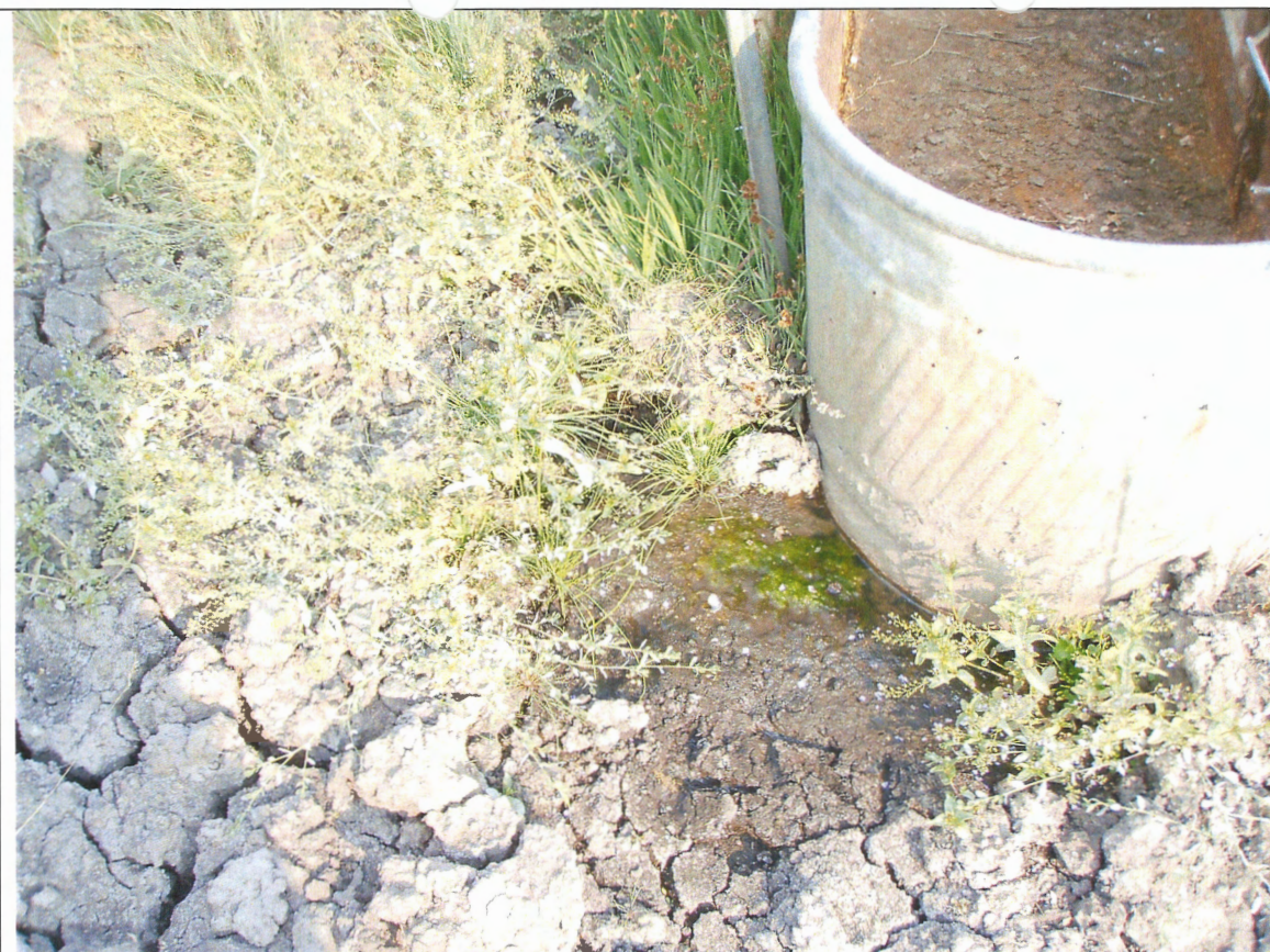
Figure 3. Shotgun BB holes in stock water tank causing water to leak out below tank.
