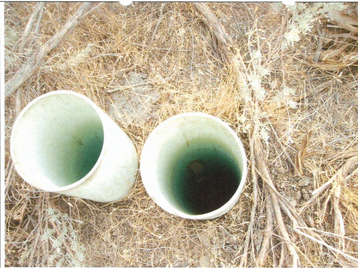
Figure 1. Valve access between stock water and irrigation.
