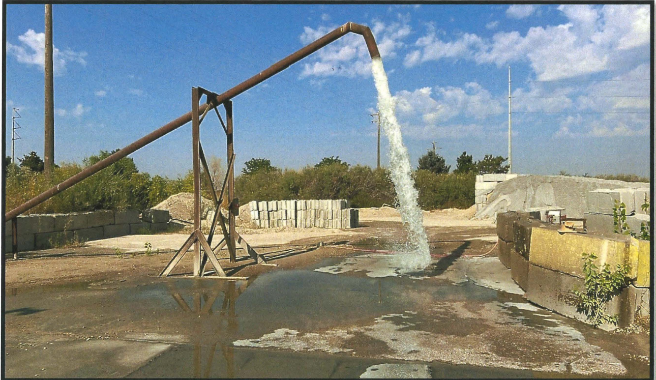
Photo 4 (below) Truck wash metering system being manually activated for demonstration.
