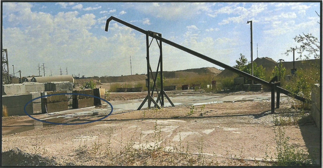
Photo 3 – Near the northwest shore of the storage pond taken facing east. The signal hose attached to the timer switch is circled on the left center of the image.
