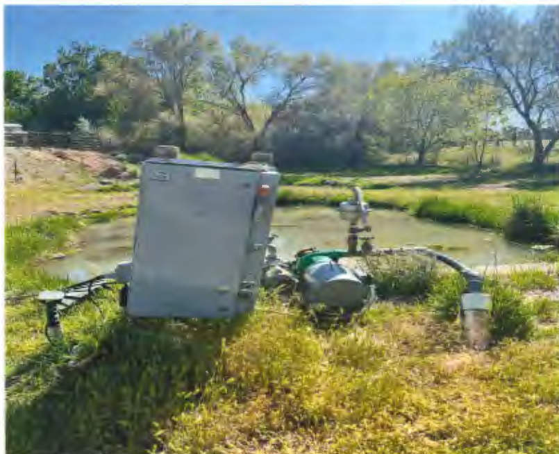
Fig. 3 Location of pump to divert irrigation water from flow through pond 2. Located in the SWSW QQ. View looking E.
