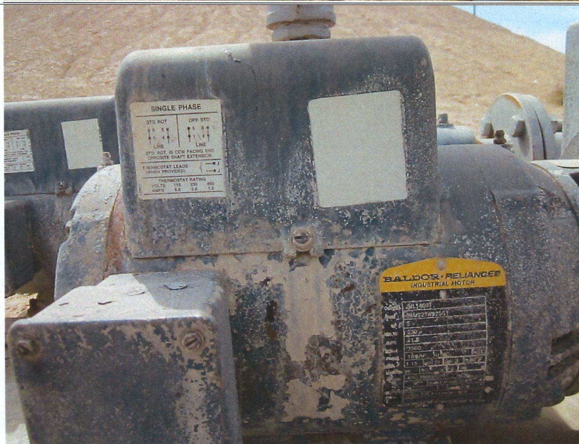
Figure 8. Baldor-Reliance 5 hp booster pump.
