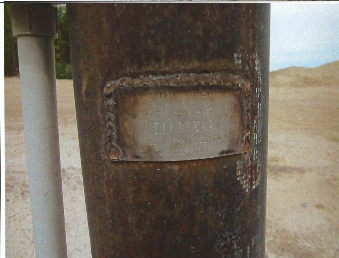
Figure 2. Well #D0060358 is a 6" well drilled for irrigation purposes on 4/13/2012. The well is 310 feet deep with the pump set at 210 feet.
