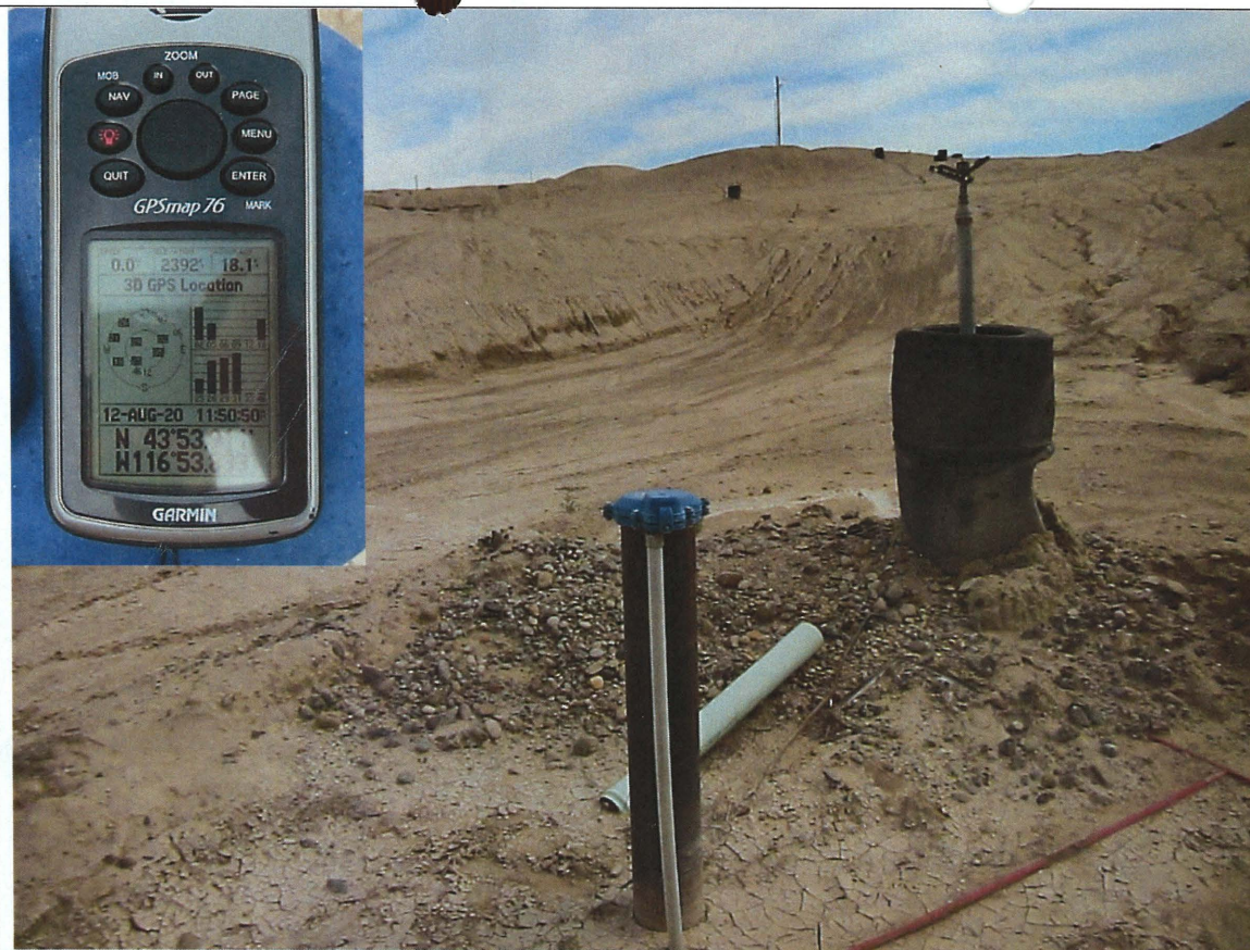
Figure 1. Well head located at 43°53.911'N, 116°53.833'W is the point of diversion. The water right holder asserted that the pump is a 2.5 hp Goulds pumping 25 gpm.
