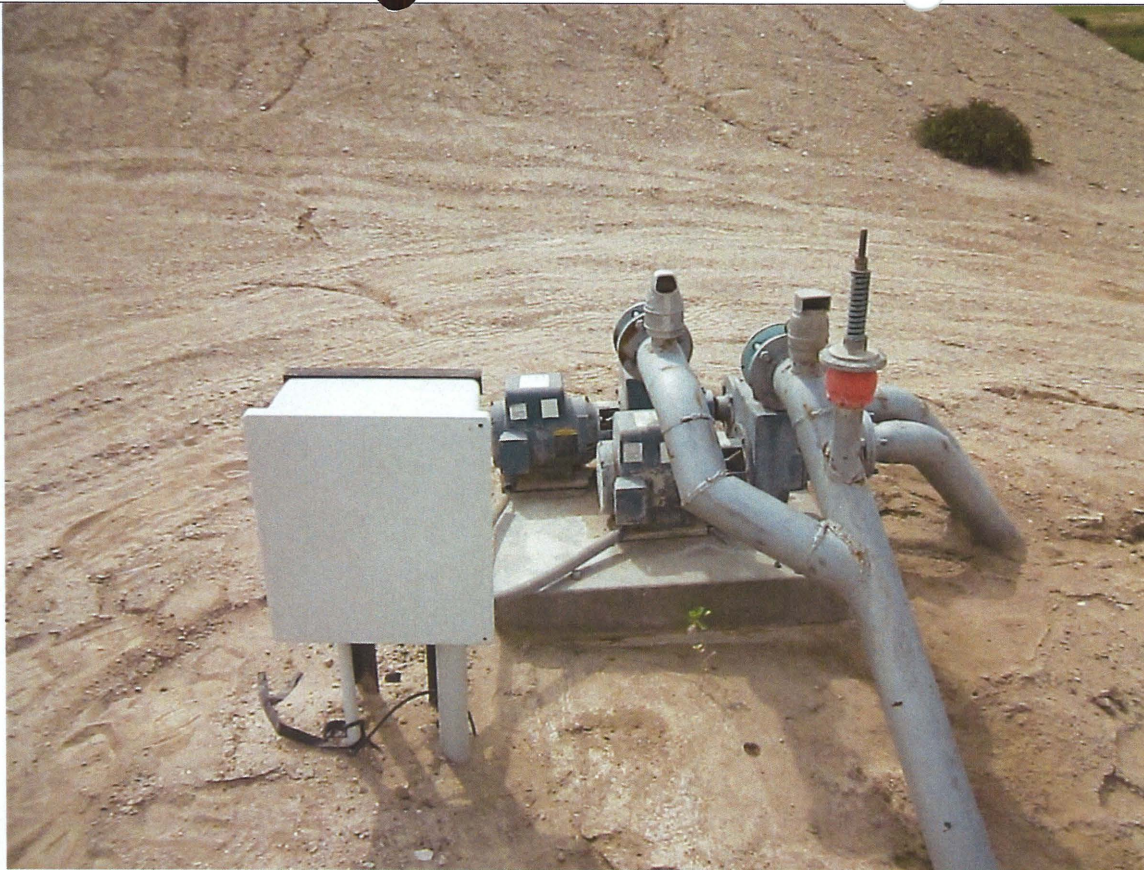
Figure 7. Two Baldor-Reliance 5 hp booster pumps distribute water to system.
