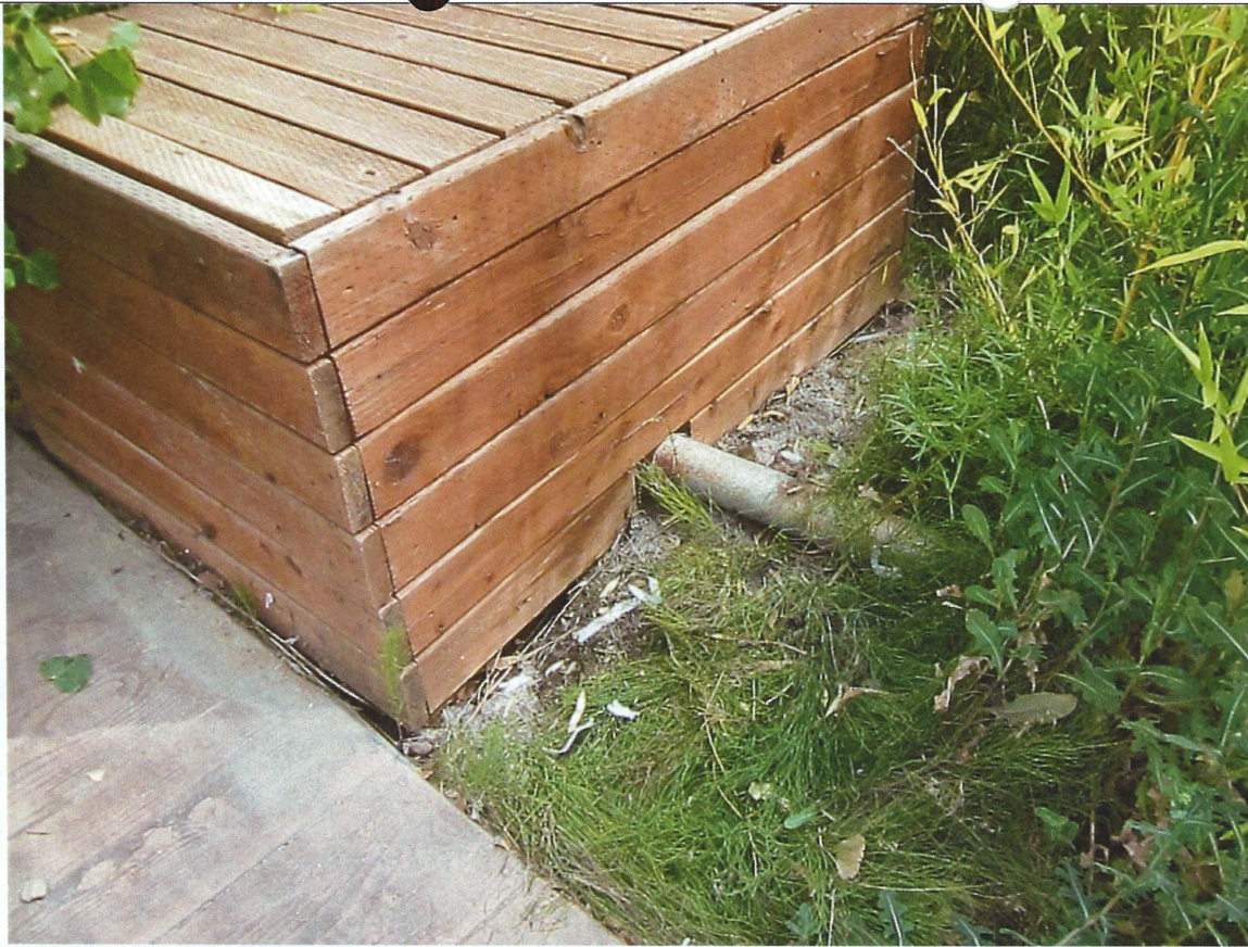
Figure 5. Pump shelter next to pond with 2" pipe exiting box.
