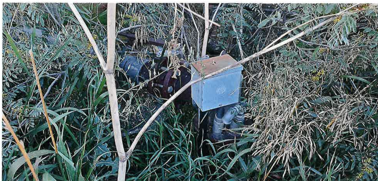
Figure 2: Close up of well head with no pump motor attached
