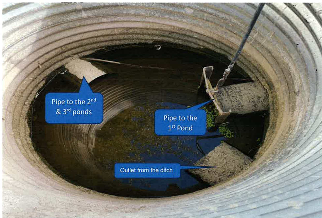
Above: Standpipe receives water from the delivery ditch, for the ponds
