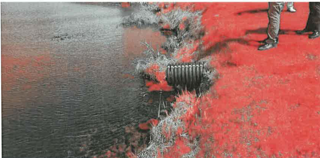
Pipeline discharge for Settlers and Well 1 water to Pond 1.
