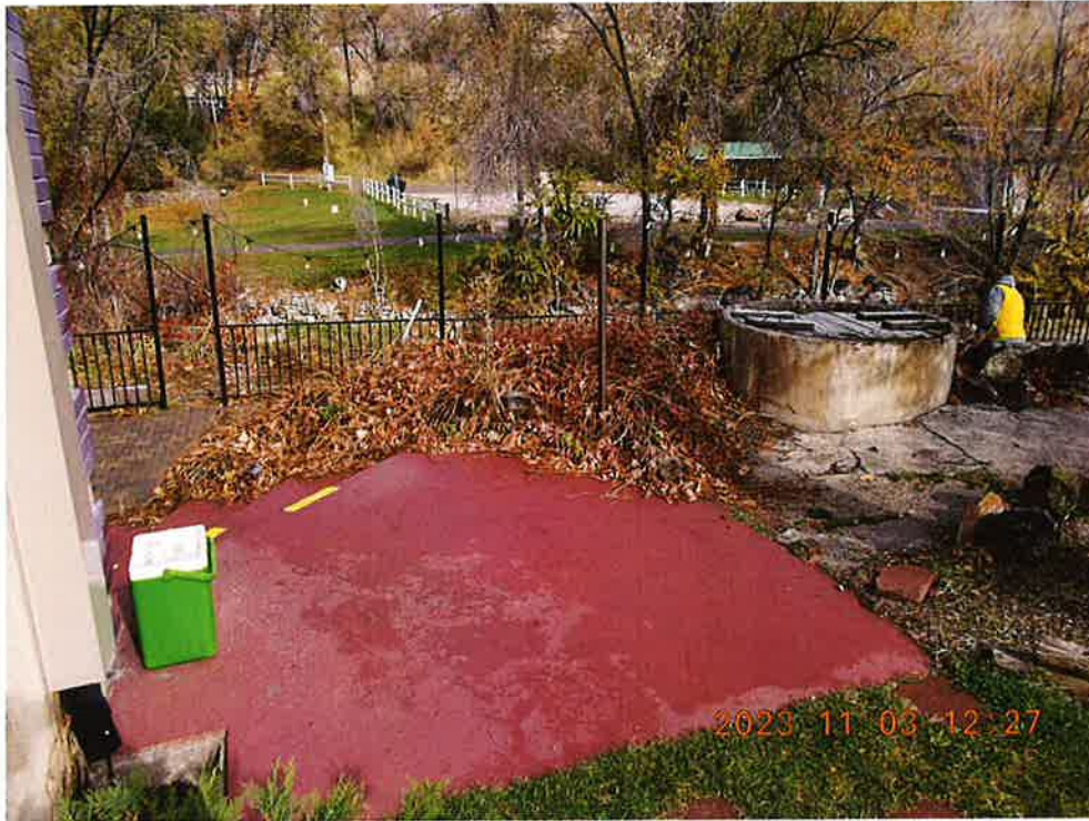
Photograph 1. Geothermal well, viewing northwest.
