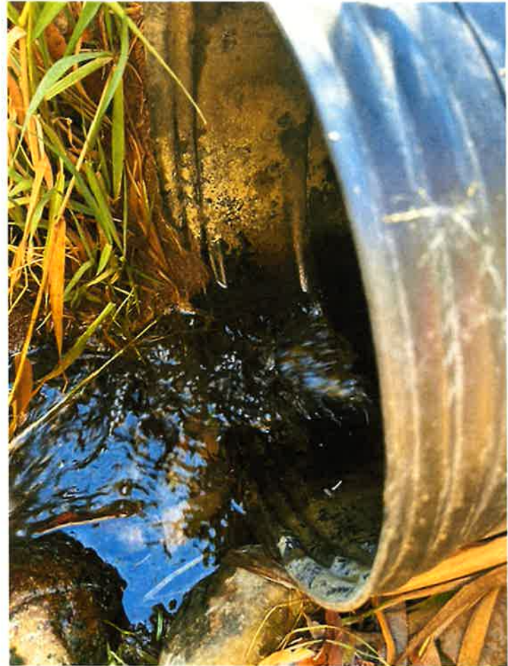
Outflow pipe with marks confirming much higher flow.
