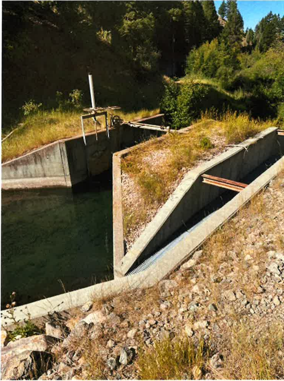
Georgetown Irrigation Company Diversion on Georgetown Creek Center of photo is headgate. Right side of photo is inoperable fish ladder.
