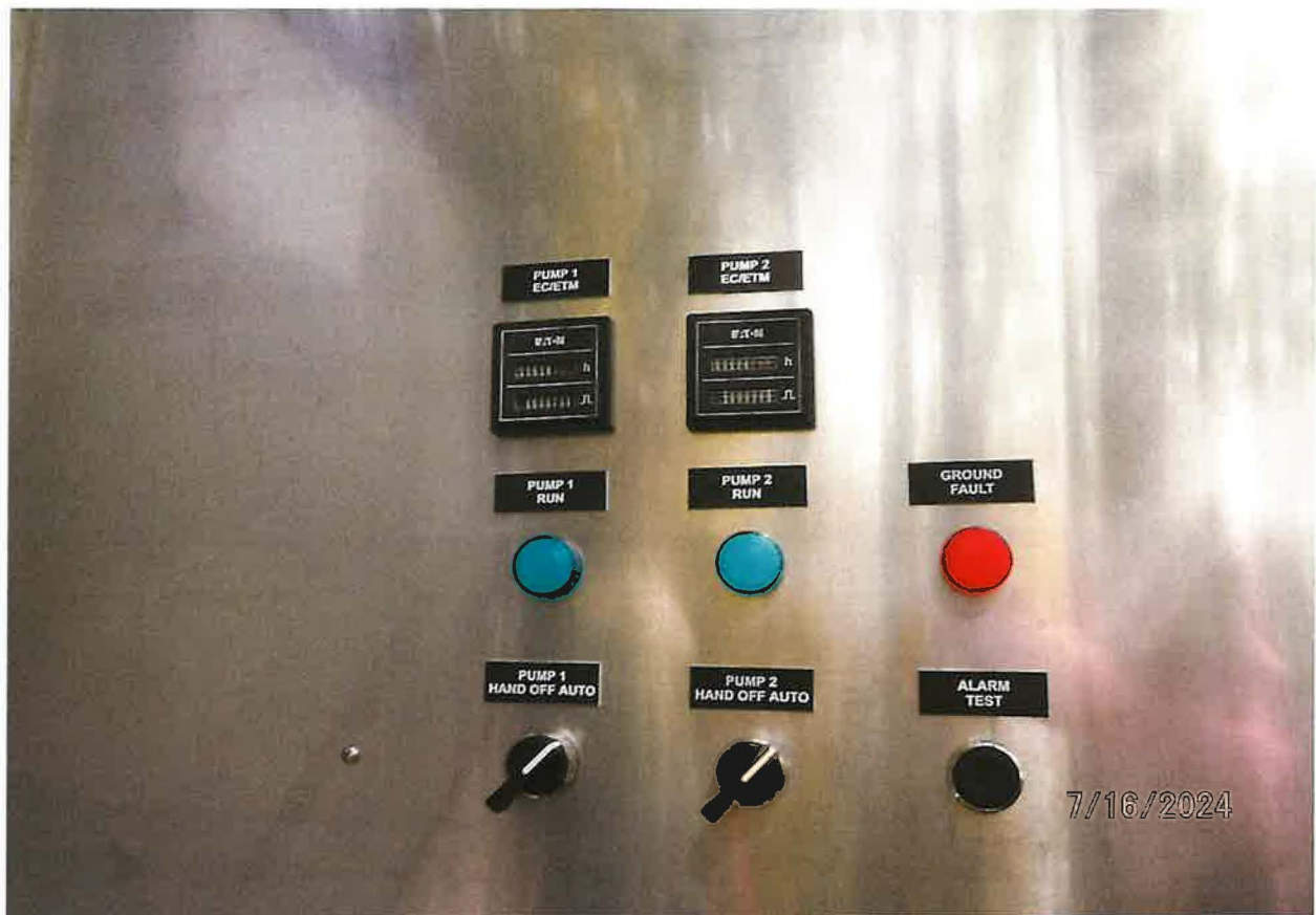
DIVERTING WORKS – PUMP CONTROL PANEL – LOCATED NEAR SHORE LINE ON ACCESS ROAD
