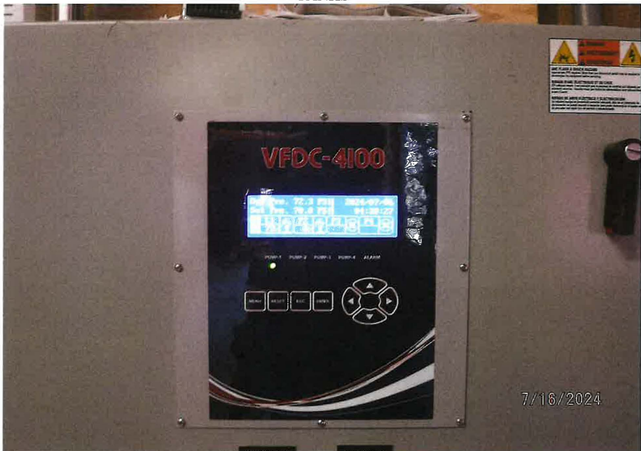
SJE RHOMBUS CONTROL PANEL WITH 75 PSI OPERATING PRESSURE OF PRESSURE TANKS SERVE AS PUMP CONTROLS FROM STORAGE TANKS (24HR IMPOUNDMENT)
