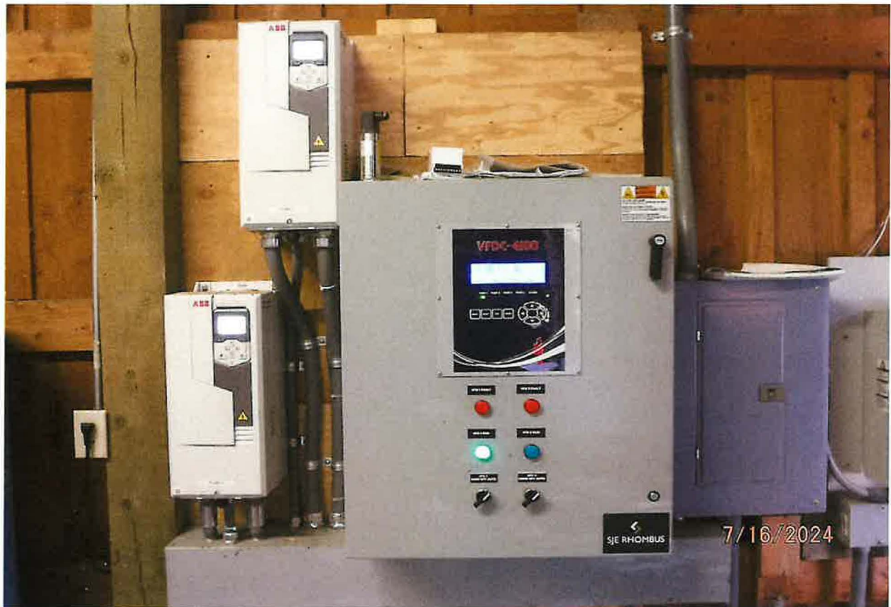
BOOSTER PUMP(S) CONTROL PANEL LOCATED WITHIN SHOP NEARBY STORAGE TANKS
