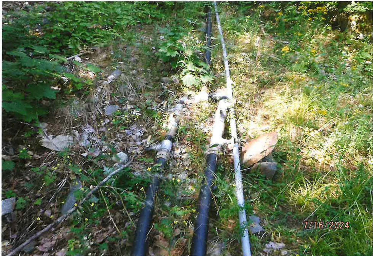
TWO INTAKE PIPES NECKING DOWN TO A SINGLE POLY-PIPE LINE
