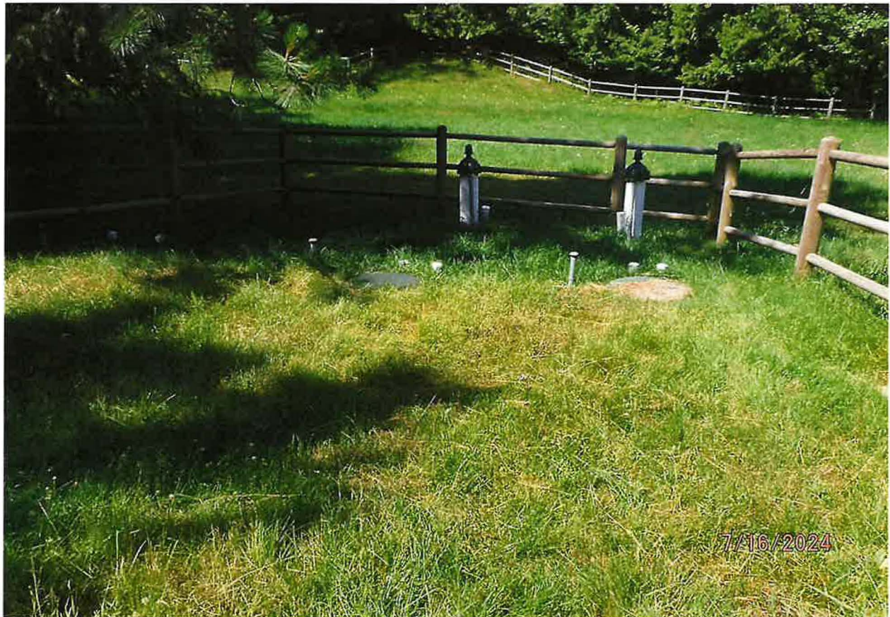
3-EACH 1,500 GAL STORAGE TANKS WITH 7.5 HP BOOSTER PUMPS USED TO DISTRIBUTE WATER TO IRRIGATION POU
