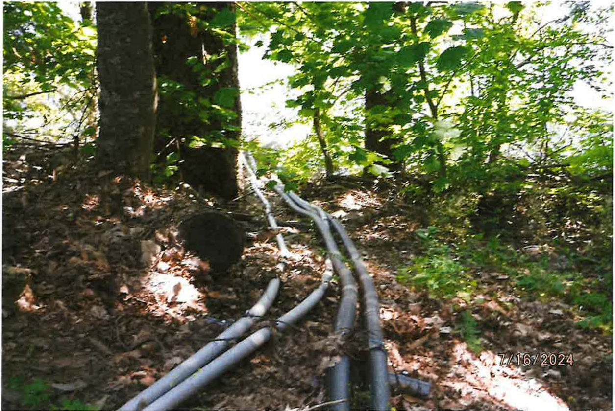
CONVEYANCE SYSTEM – 2 EA POLY-PIPE INTAKE LINES SET UP TO USE PUMPS IN A LEAD-LAG NORMAL OPERATION CONVERGING TO A SINGLE PIPELINE ROUTED UP-GRADE TO STORAGE TANKS PRIOR TO IRRIGATION DISTRIBUTION
