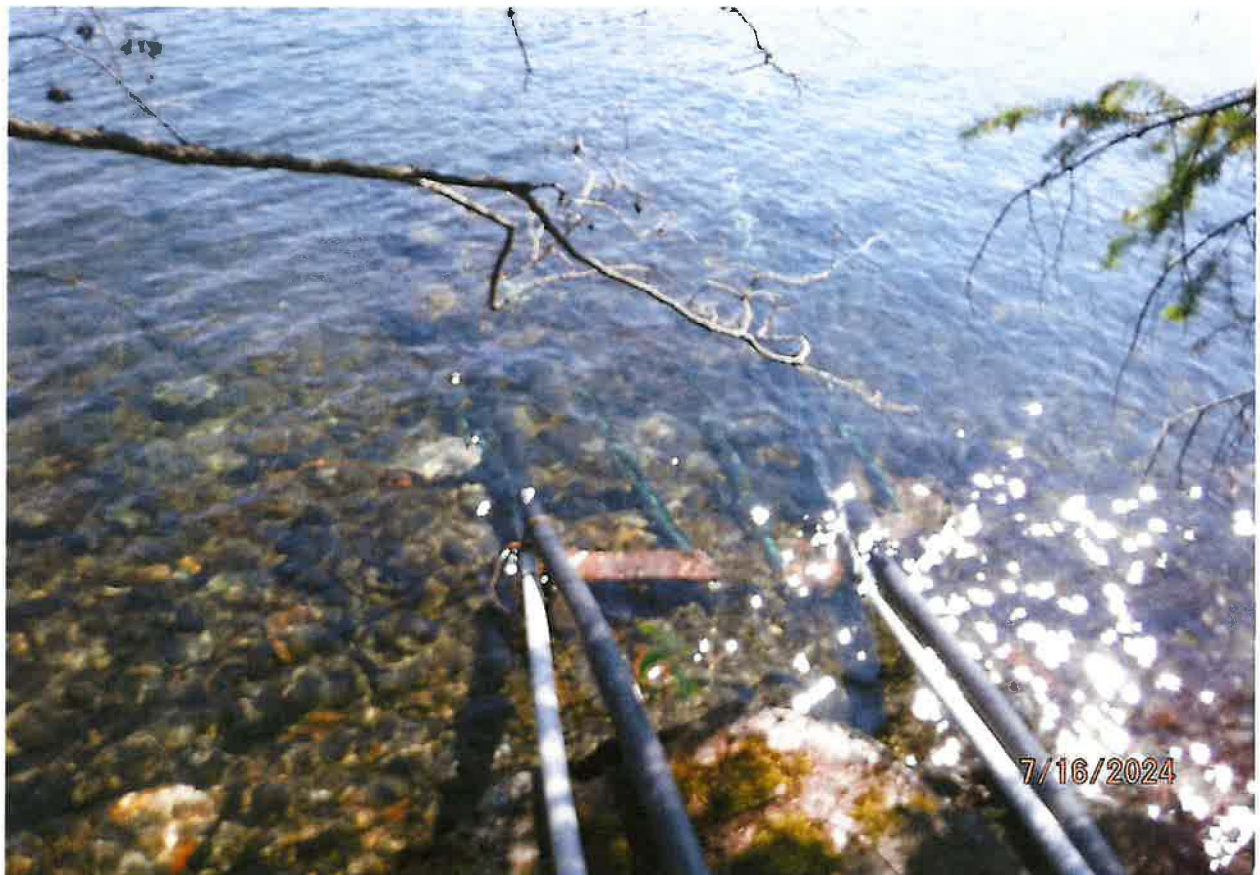
POD – 2EA INTAKE PIPES WITH 2EA SUBMERSIBLE PUMPS IN LAKE PEND OREILLE
