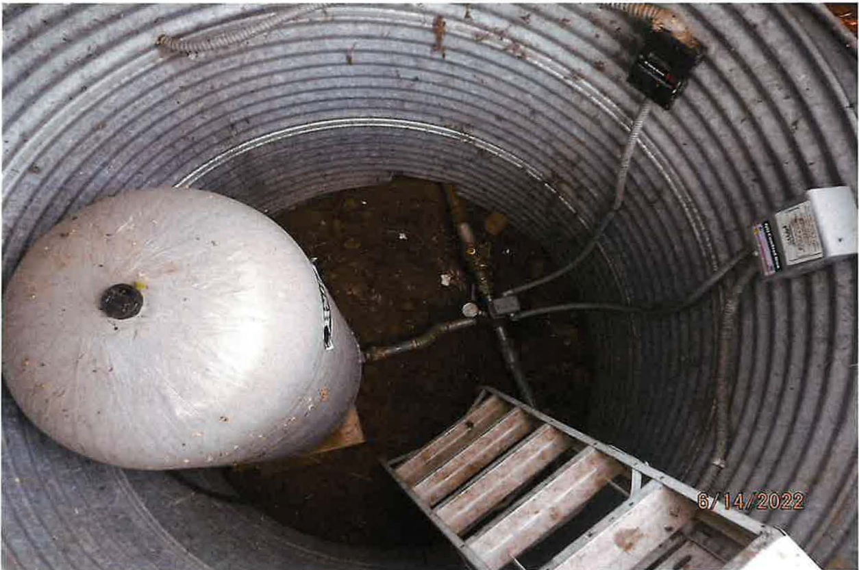
CULVERT VAULTED PUMP STATION
