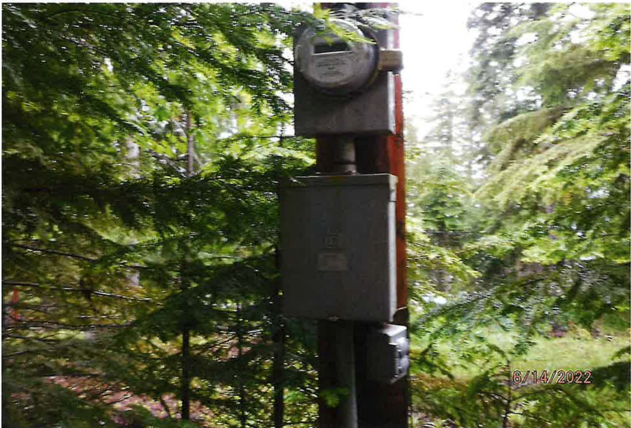
ELECTRIC POWER READER BOX
