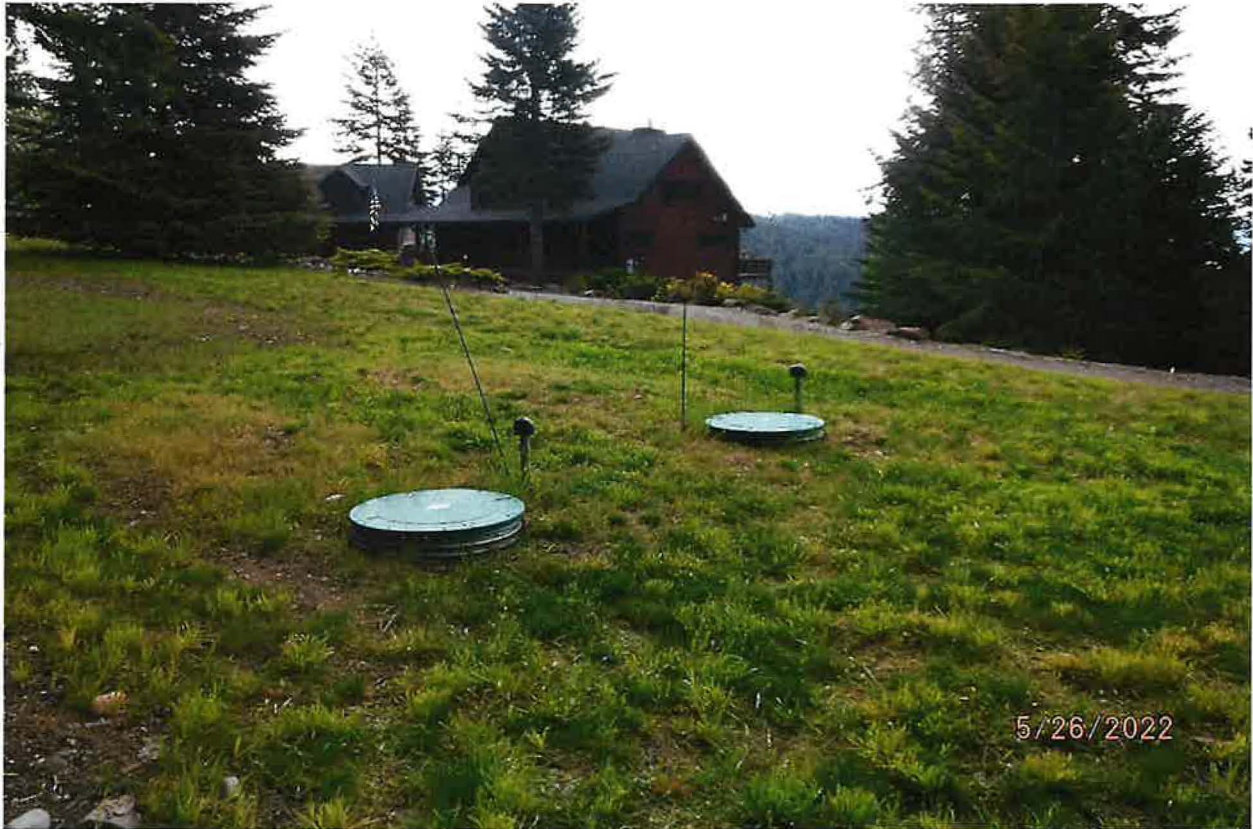
2EA 3,000 GALLON COMMUNITY STORAGE TANKS INCLUDED IN WATER CONVEYANCE SYSTEM
