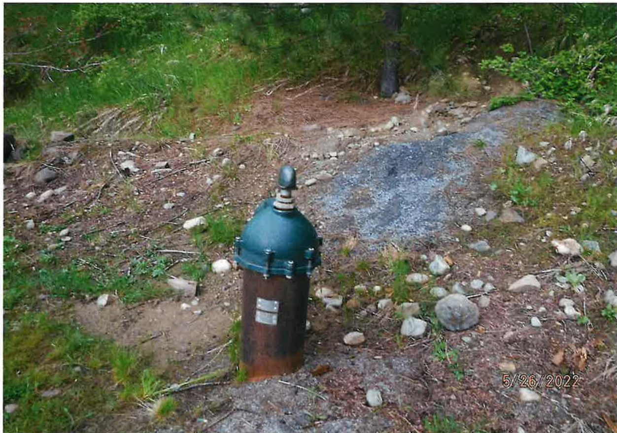
GROUNDWATER POD – WELL D0076649 & D0079009; NORTHERN MOST WELL THAT HAS BEEN DEEPENED.
