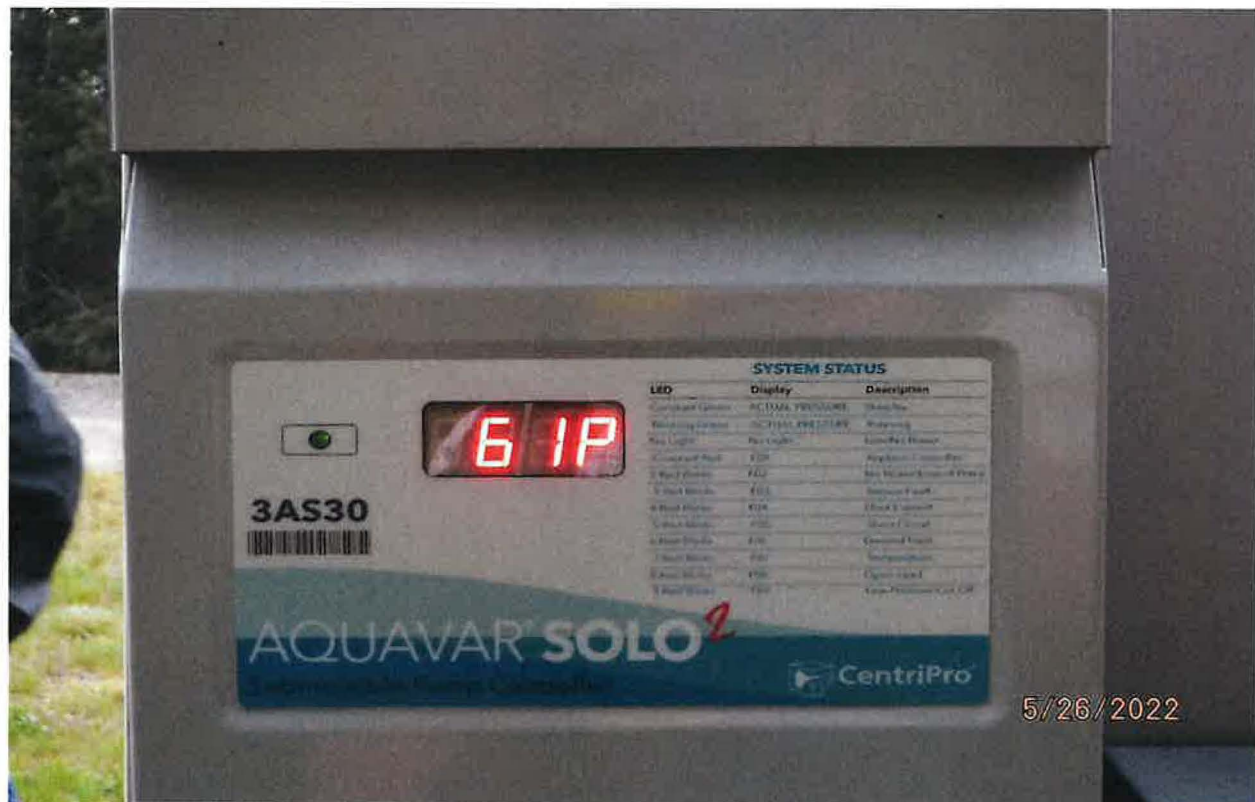
61 PSI WATER SYSTEM OPERATING PRESSURE
