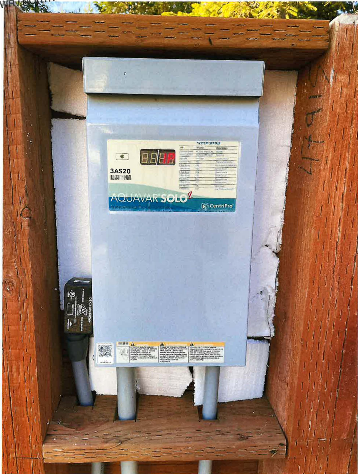
Image sent by Mr. Ted Swanstrom by email received on 6/12/2023 – illustrates the pump motor control panel.
