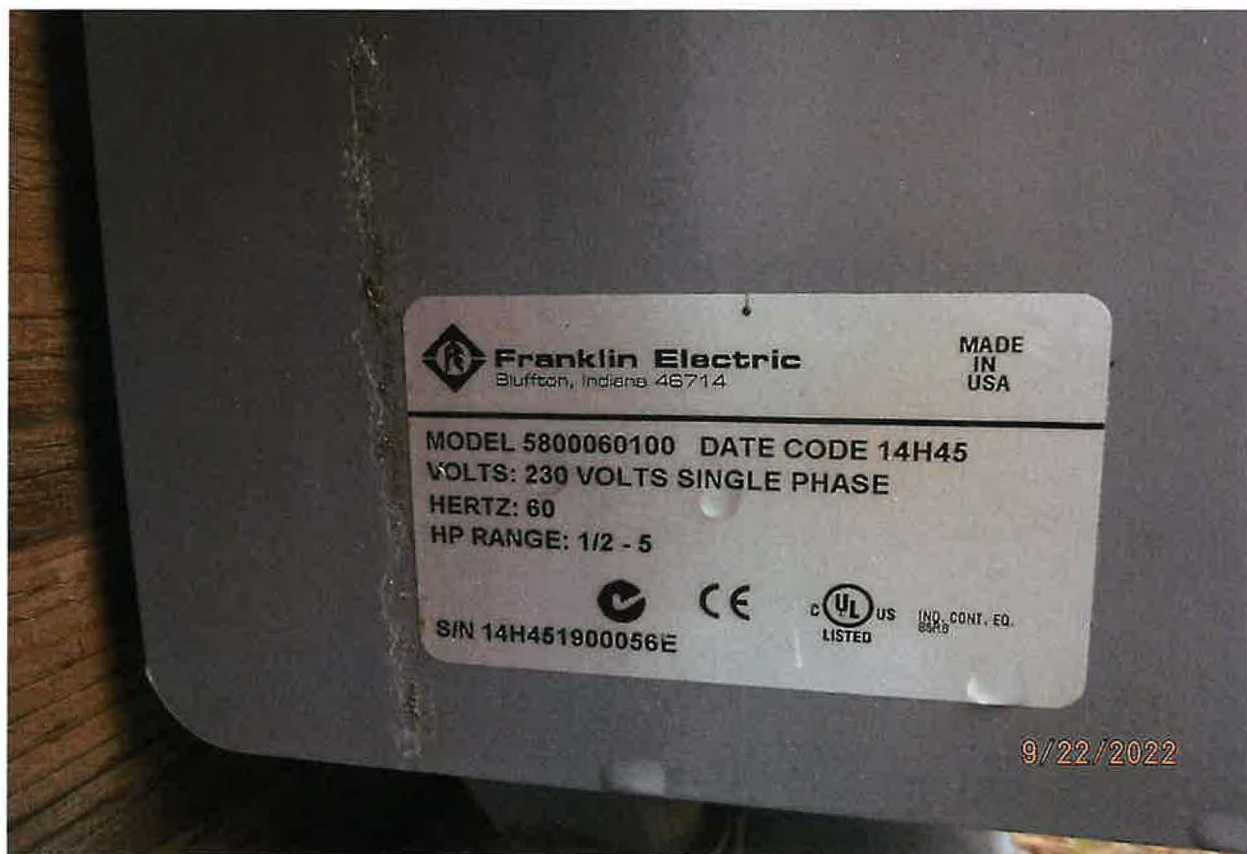
1.5 HP PUMP WITH \frac{3}{4} HP MOTOR (VFD) TRANSFER PUMP INSTALLED IN STORAGE TANK
