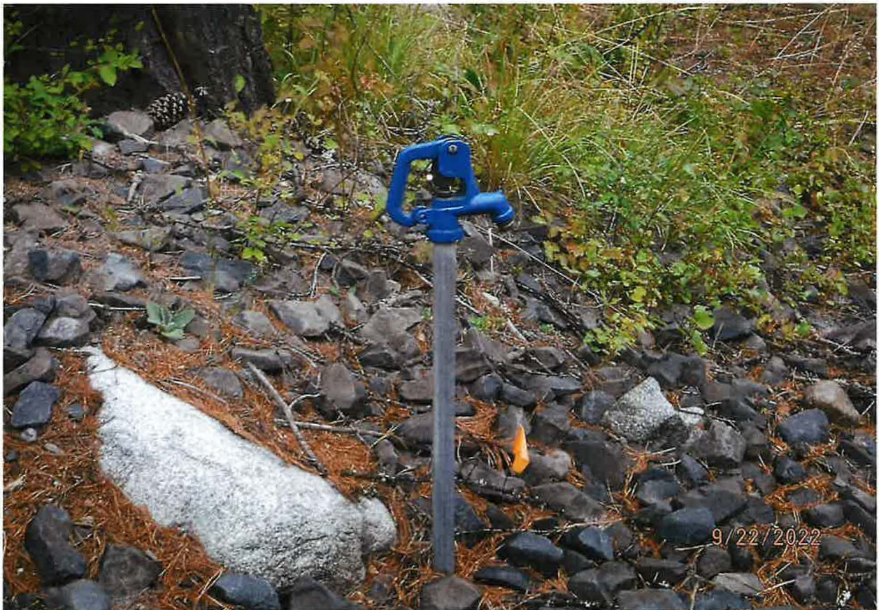
FROST FREE HYDRANT FOR LT1, BLK1 WHERE HOME SERVICE LINE STUBS INTO WATER MAIN
