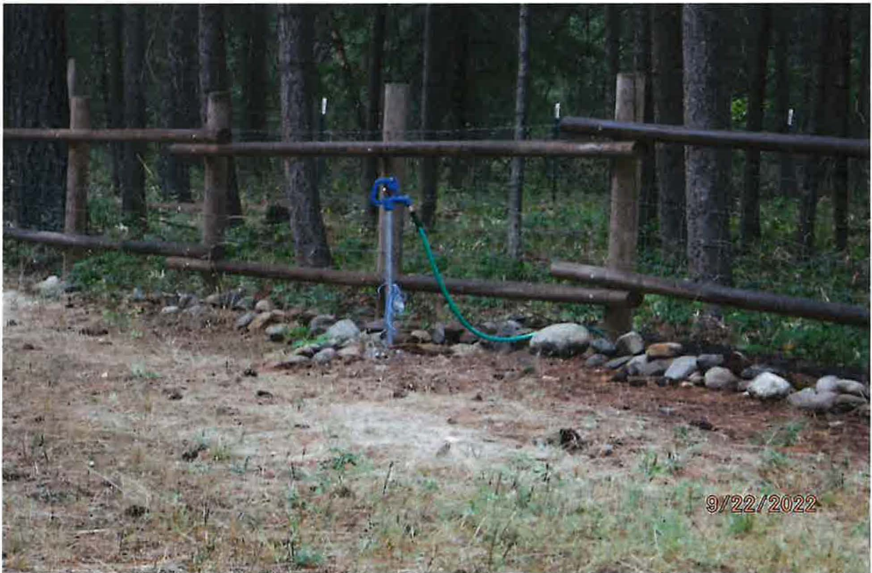
FROST FREE HYDRANT FOR LT3, BLK1 WHERE HOME SERVICE LINE STUBS INTO WATER MAIN
