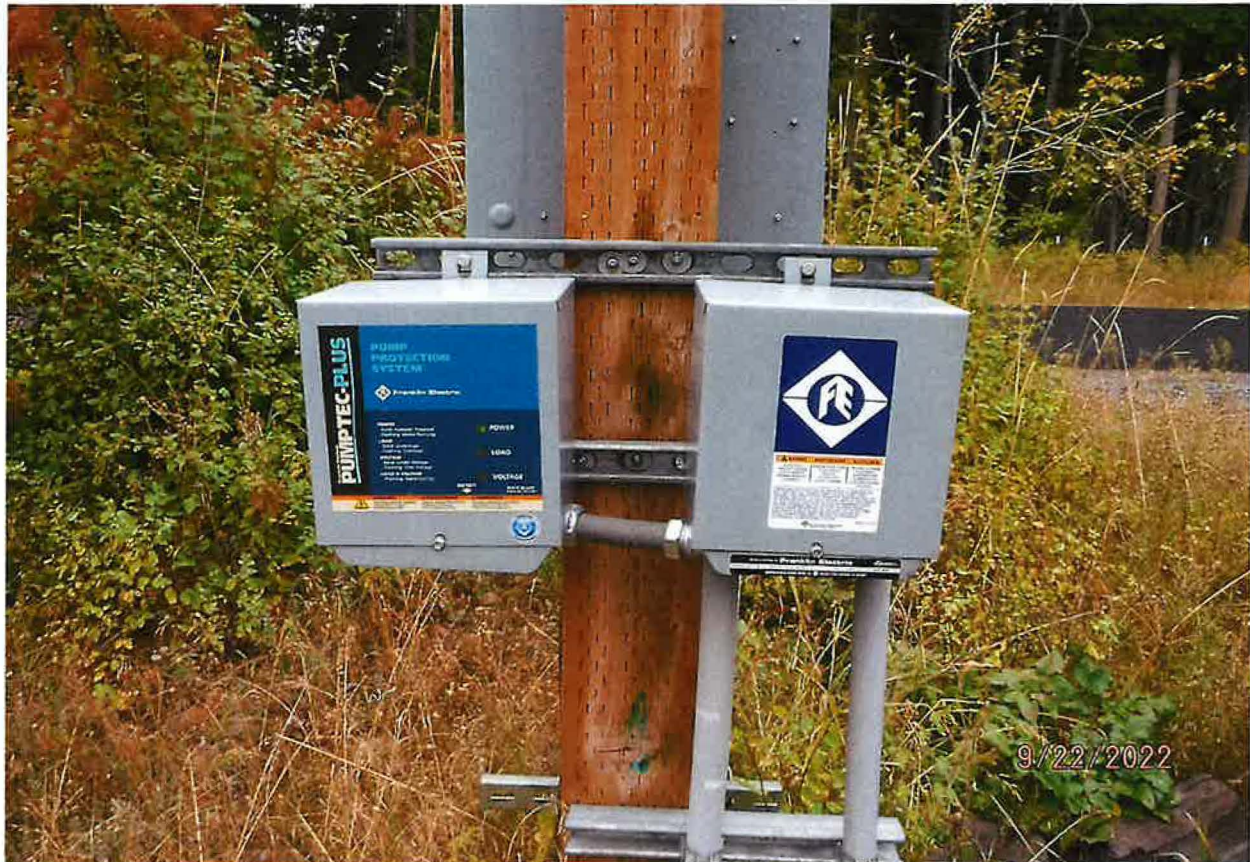
CONTROL PANELS FOR D0069867
