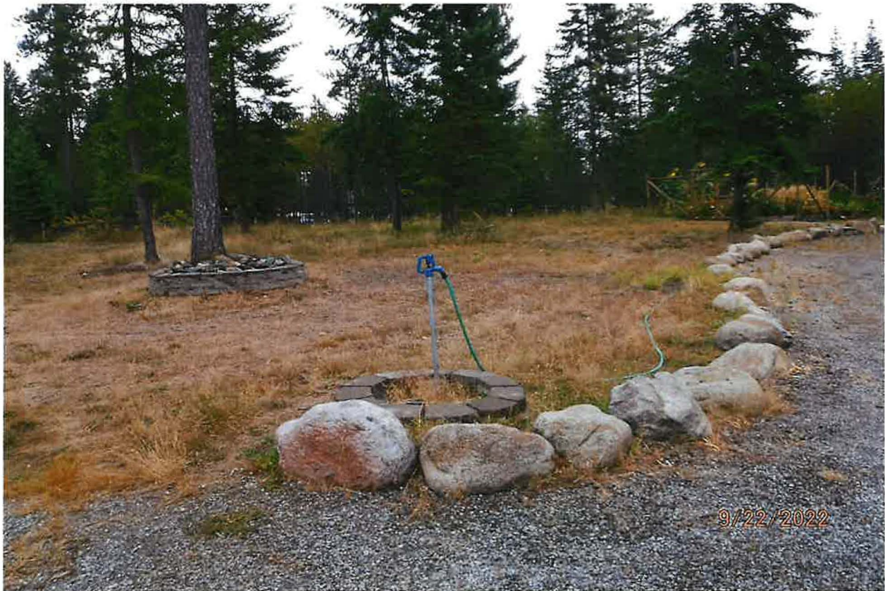
FROST FREE HYDRANT FOR RP53N02W193400 WHERE HOME SERVICE LINE STUBS INTO WATER MAIN
