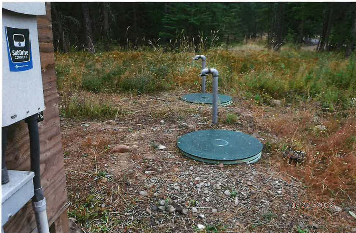
2 STORAGE TANKS IN COMMUNITY SYSTEM – SIZE UNKNOWN
