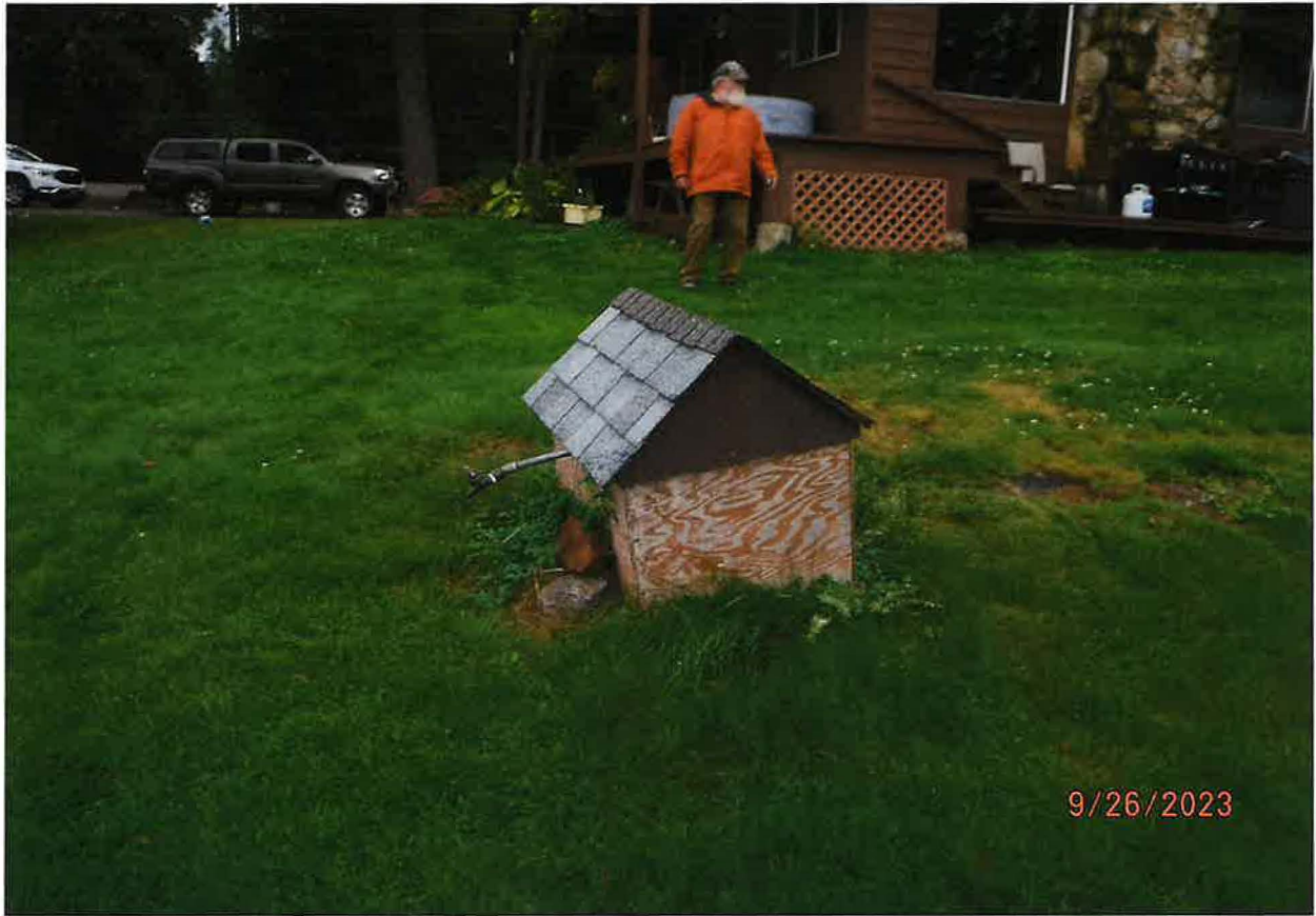
BURIED POLY LINE TO SMALL DOGHOUSE CONTAINING WATER TRANSFER PUMP
