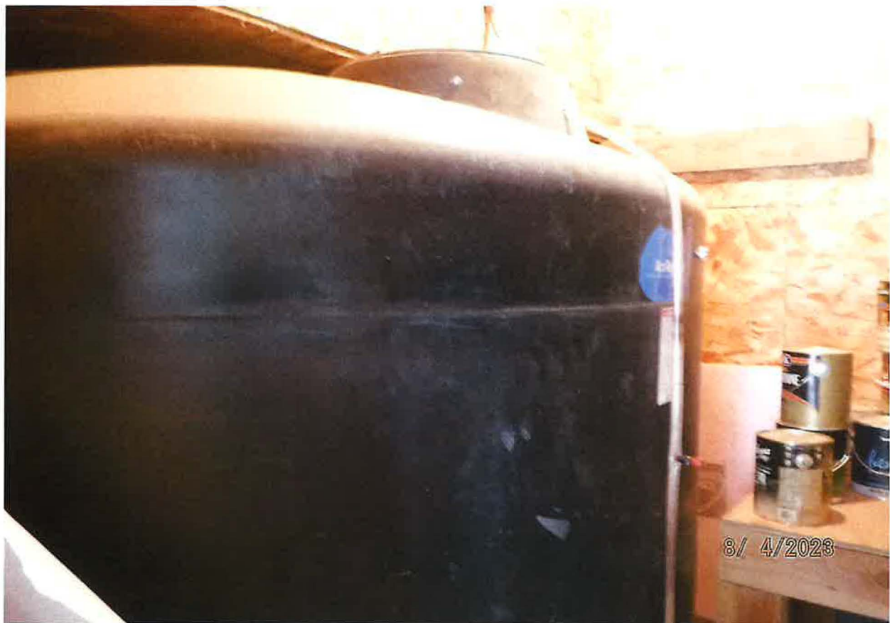
1,000 GAL STORAGE RESERVOIR LOCATED INSIDE SHOP
