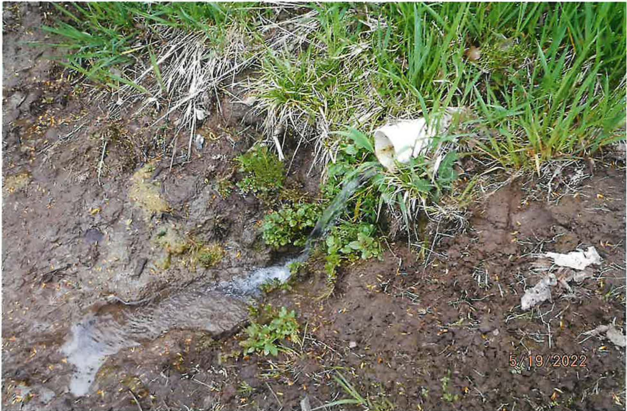
POD – SPRING #2 SPRING BOX AND DIVERSION TO STORAGE COMPONENT. SPRING CO-LOCATED WITH POND
