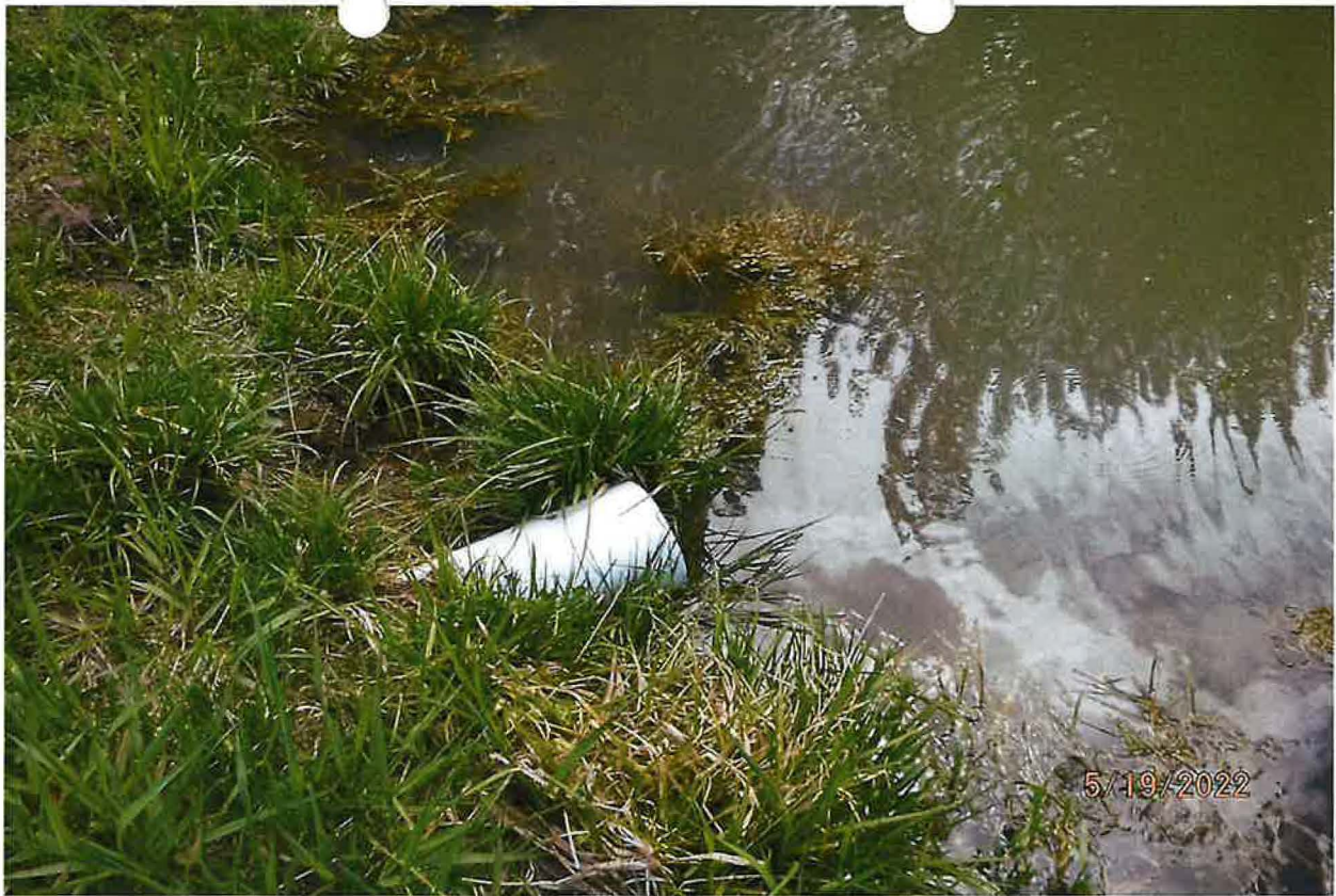
OVERFLOW DEVICE – 6 INCH PVC PIPE ON EAST SIDE OF POND ALLOWS WATER TO CONTINUE DOWNSTREAM
