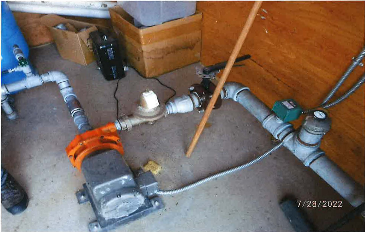
BOOSTER PUMP INSTALLED IN DIVERSION WORKS FOR WELL D0072232 – NEVER BEEN TURNED ON, INTENDED FOR USE IN EVENT FIRE SUPPRESSION IS REQUIRED.
