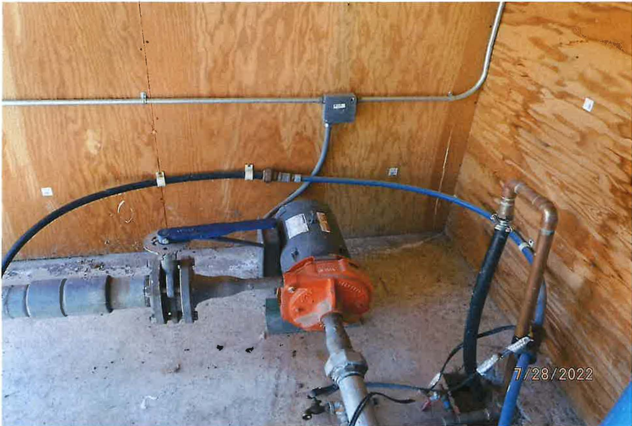
CENTRIFUGAL BOOSTER PUMP (NEVER BEEN USED) INSTALLED ON SYSTEM FOR FIRE PROTECTION USE
