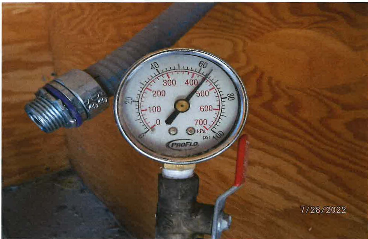
65 PSI OPERATING PRESSURE FROM PRESSURE TANKS
