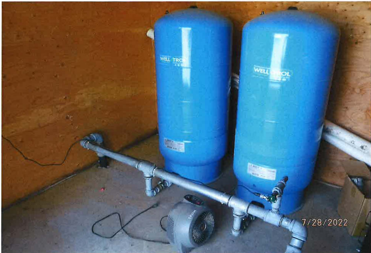
MAIN WATER LINE FROM WELL TO 2 PRESSURE TANKS BEFORE DISTRIBUTION TO IRRIGATION SYSTEM
