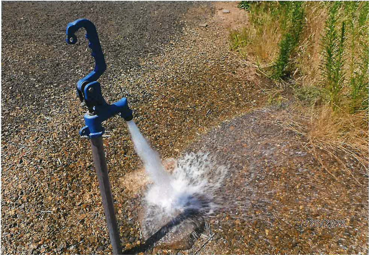
PRESSURE INDUCED FLOW FROM FROST-FREE HYDRANT CO-LOCATED WITH WELL D0072232
