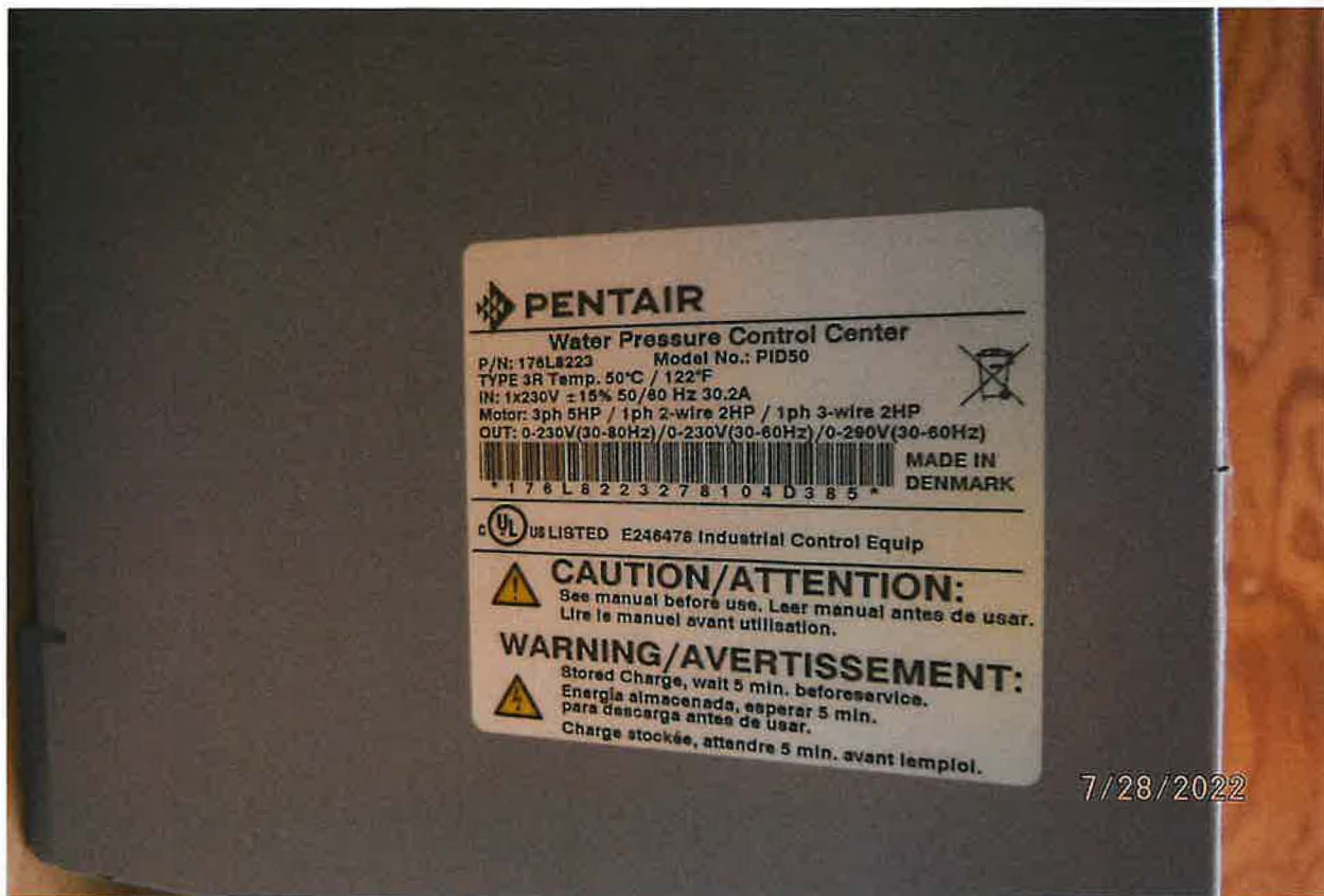
PENTAIR 5 HP 3 PHASE VARIABLE FREQUENCY DRIVE PUMP MOTOR INSTALLED IN WELL BY BUILDING
