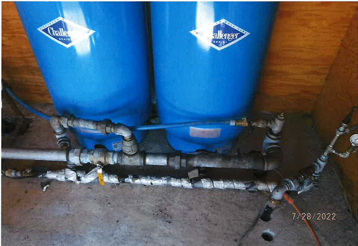
POD – WELL 95-92-N-87-100 – WELL WITH CONCRETE PAD AND PUMP HOUSE DEVELOPED OVER WELL
