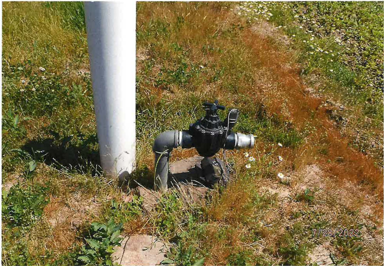
IRRIGATION RISER PIPES
