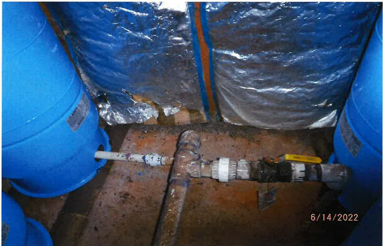
CONVEYANCE SYSTEM – PRESSURE TANKS AND MAIN SERVICE LINE OUT FROM PUMP HOUSE
