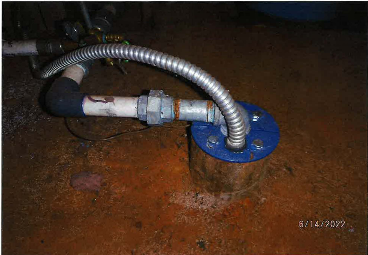
POD – GROUNDWATER WELL LOCATED WITHIN A PUMP HOUSE
