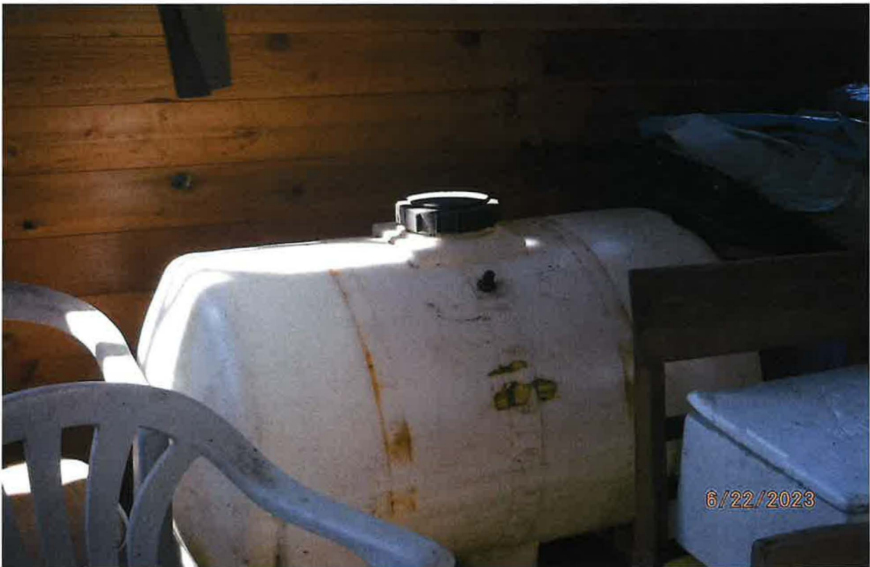
PORTABLE 250 GAL WATER TANK USED IN CABIN FOR DOMESTIC USES
