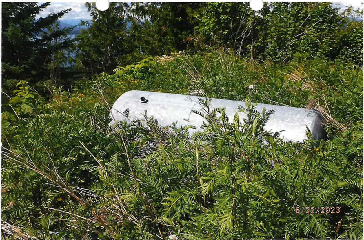
WATER TANK USED TO HOLD WATER TEMPORARILY AT CABIN LOT 7, EUREKA HEIGHTS SUB.
