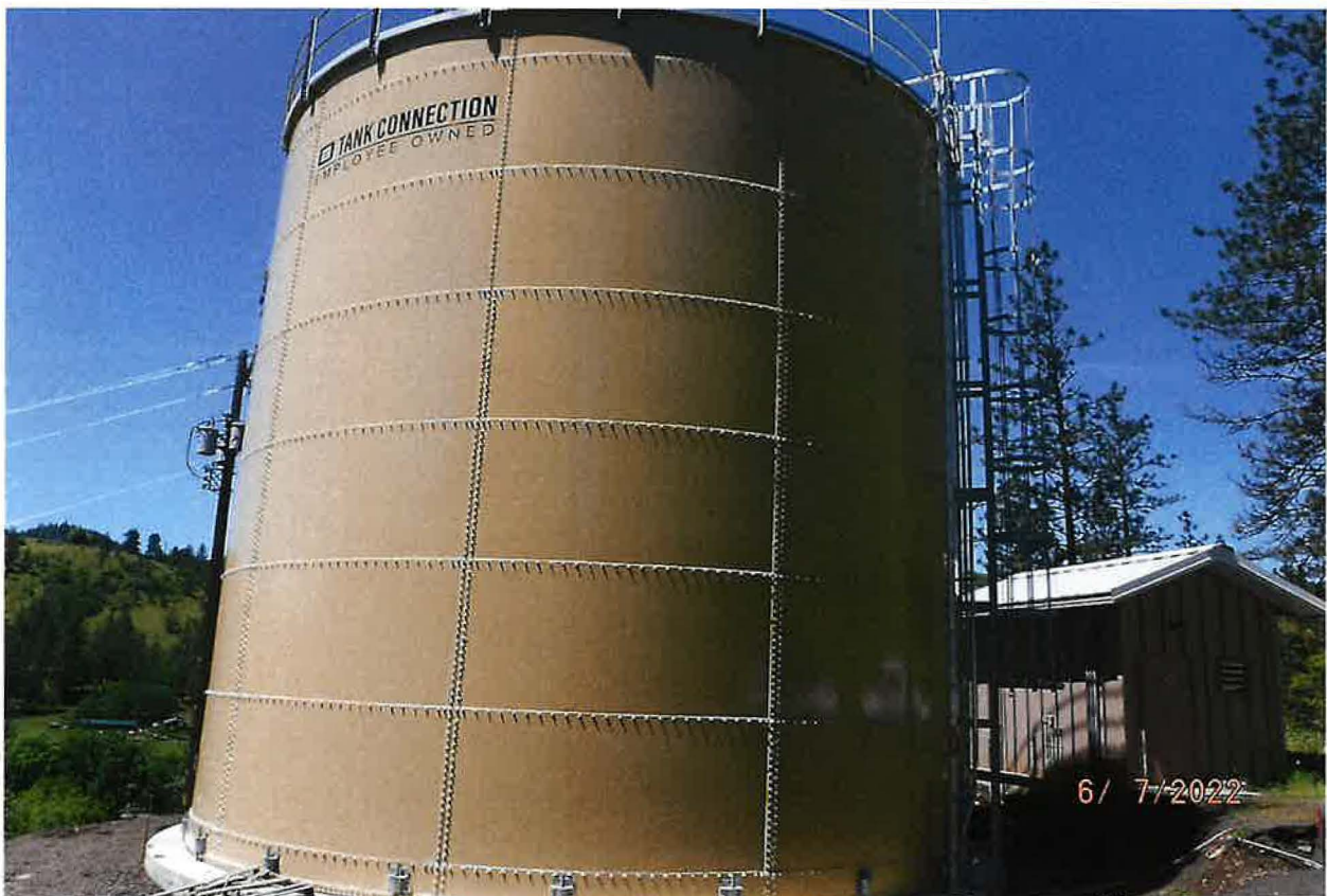
180,000 GAL STORAGE RESERVOIR, PUMP STATION WELL D0072339 IN BACKGROUND
