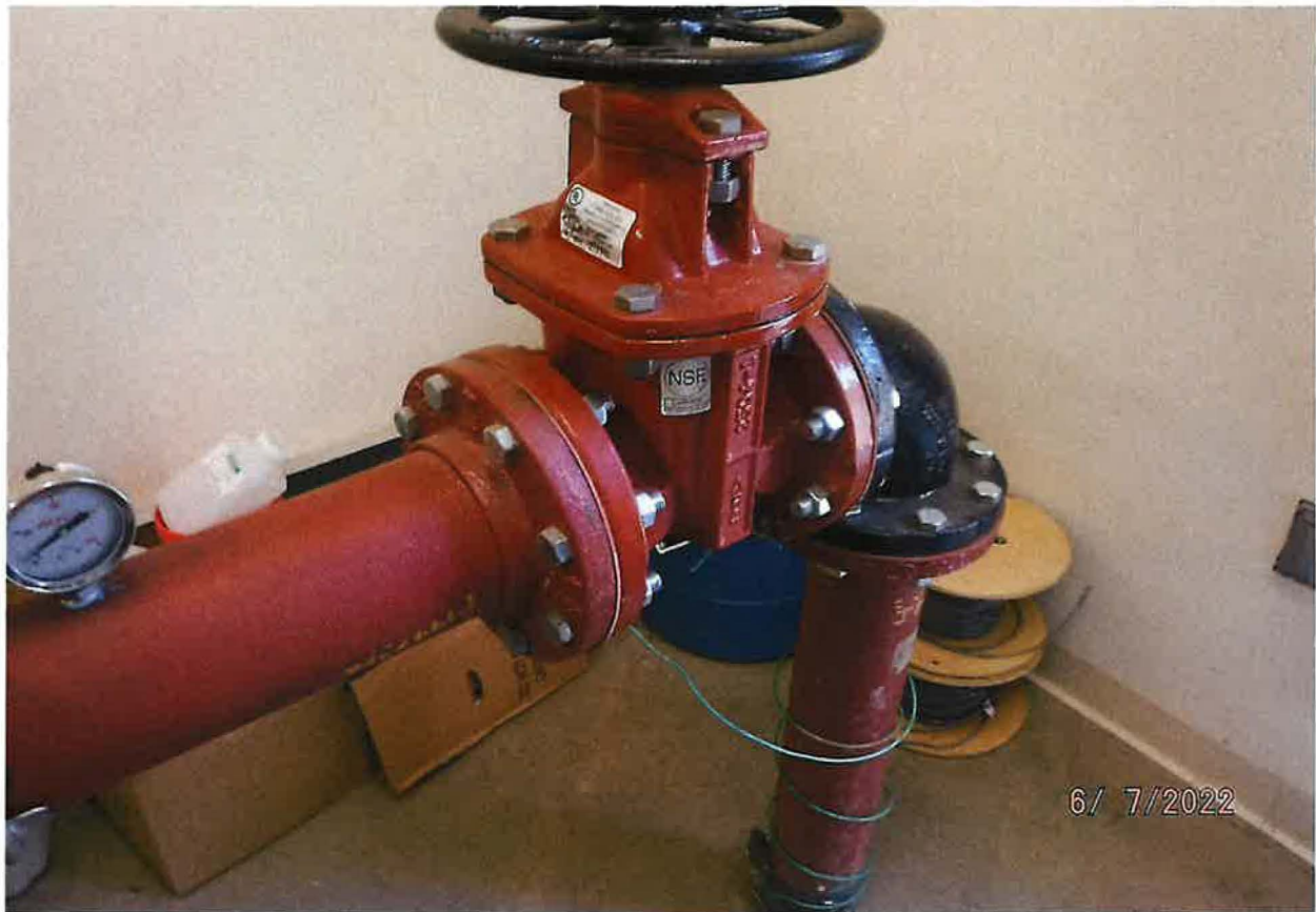
SERVICE MAIN IN FROM D0072339 TO PUMP HOUSE PRIOR TO USE
