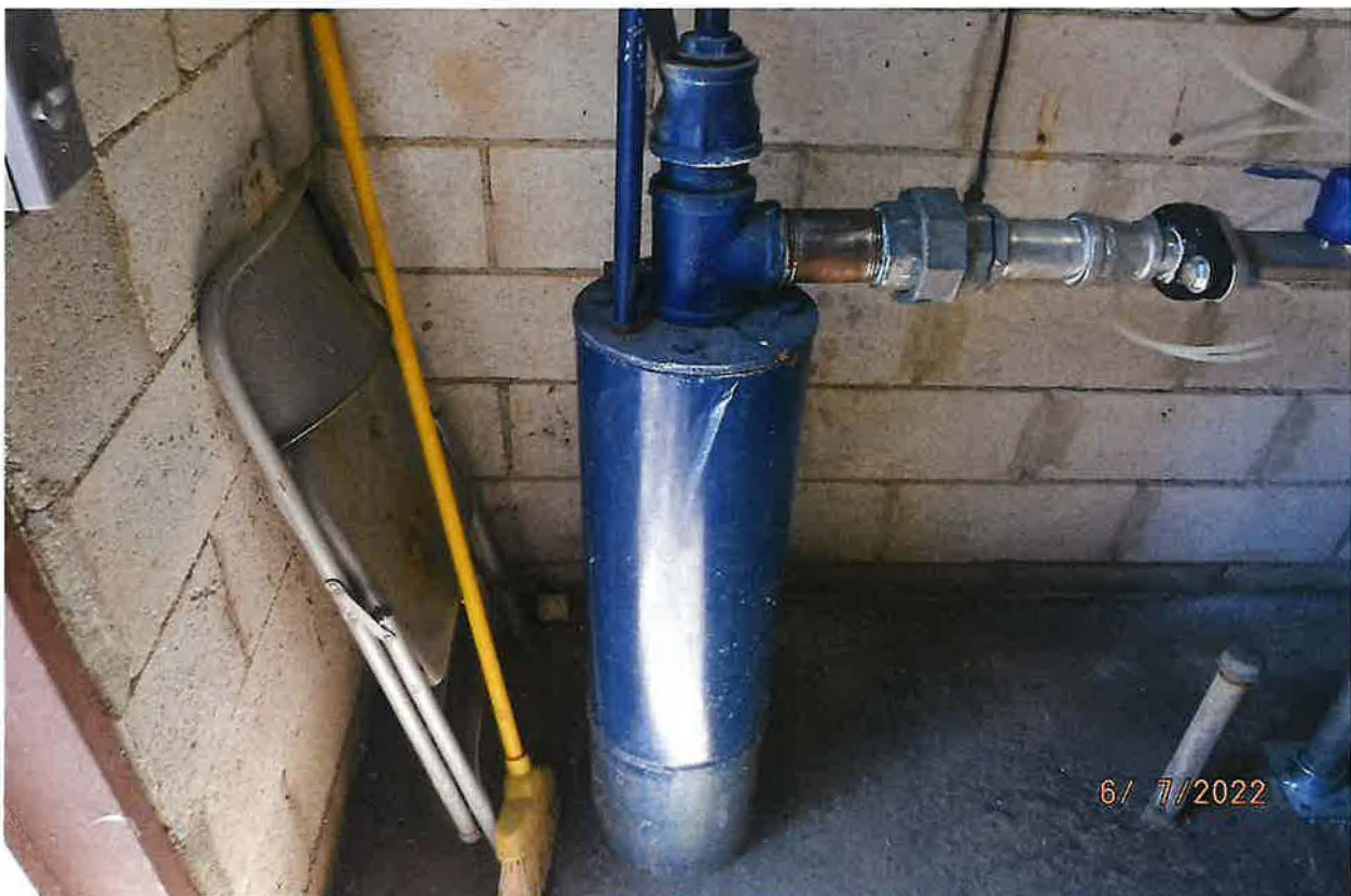
POD – GROUNDWATER WELL NE¼NE¼, SEC. 29, TWP 32N, RGE 04E
