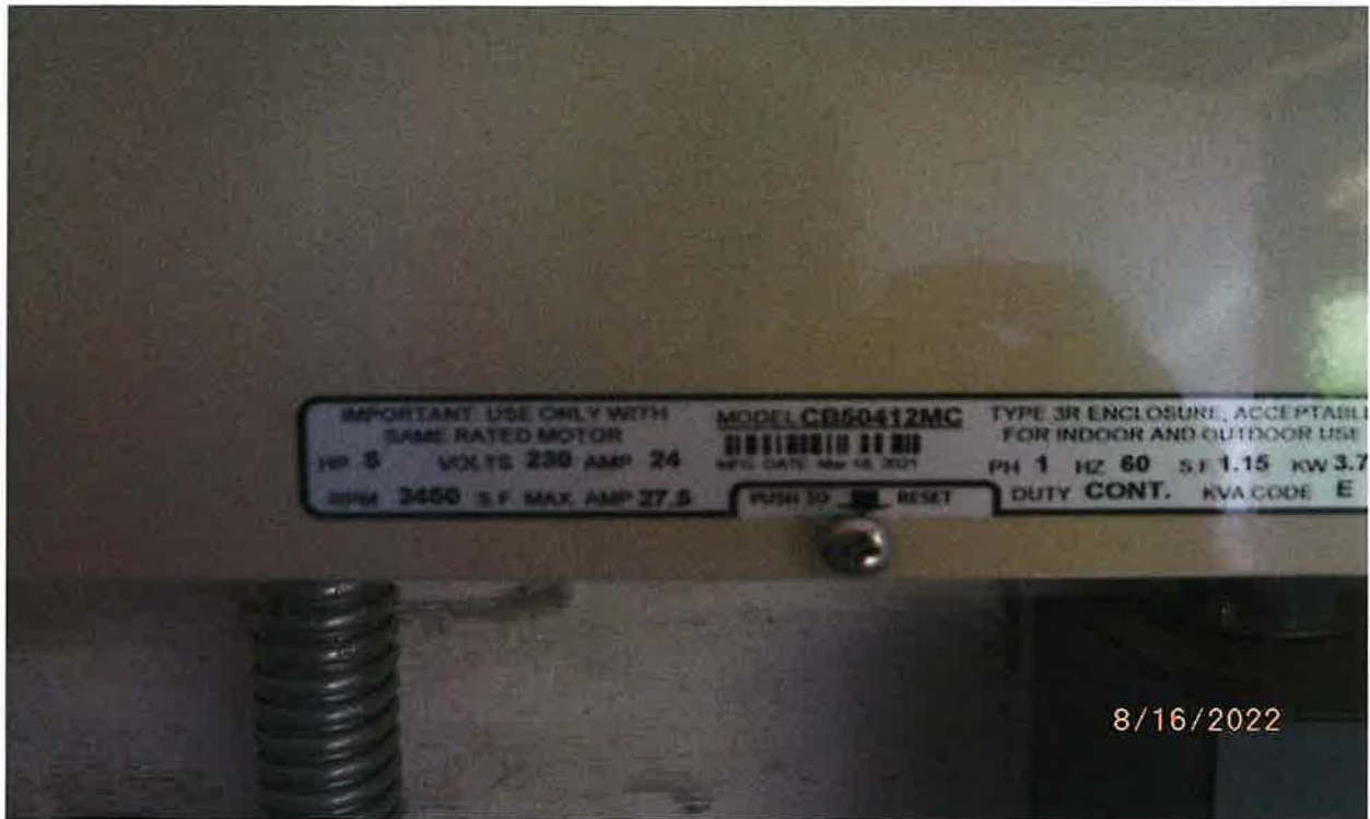
5 HP PUMP MOTOR INSTALLED IN WELL
