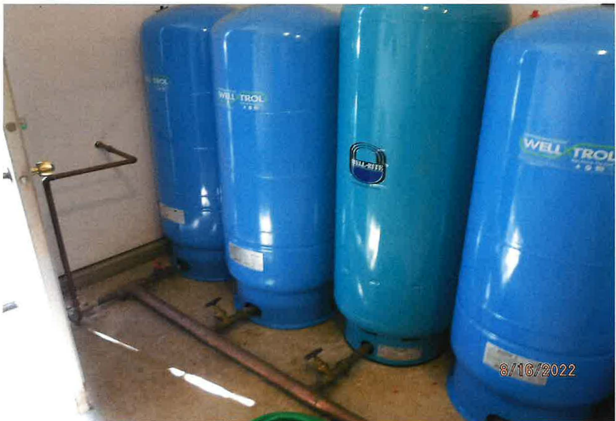
DIVERTING WORKS INCORPORATES SEVERAL PRESSURE TANKS FOR THE COMMUNITY SYSTEM
