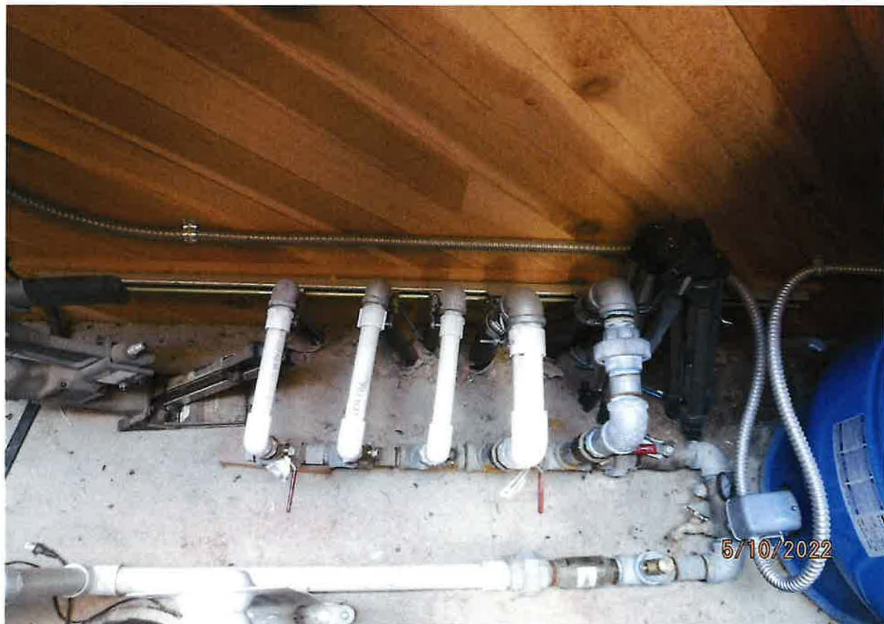
DIVERTING WORKS INCLUDES PRESSURE TANK THAT READ 45 PSI
