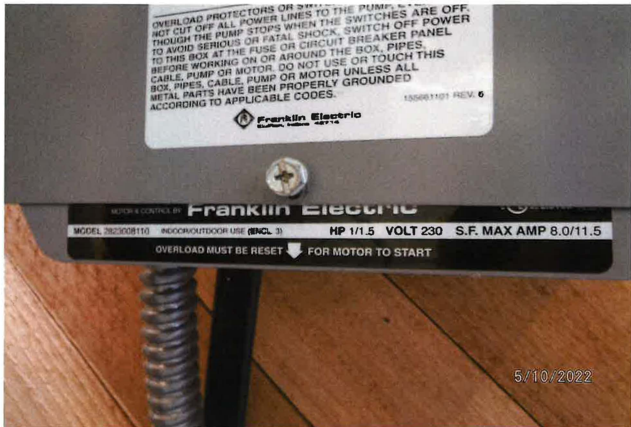
1.5 HP FRANKLING PUMP MOTOR INSTALLED IN WELL
