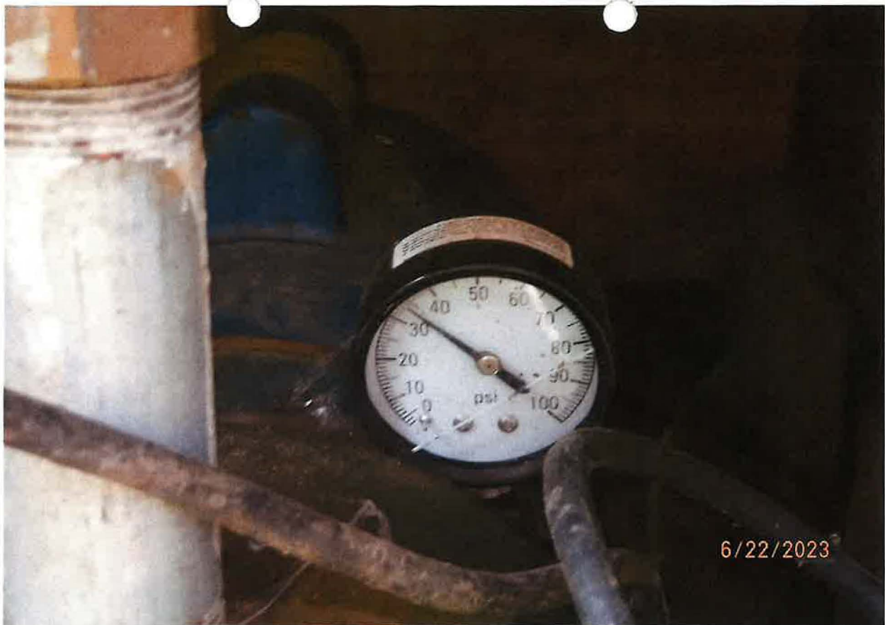
35-40 PSI IRRIGATION OPERATING PRESSURE
