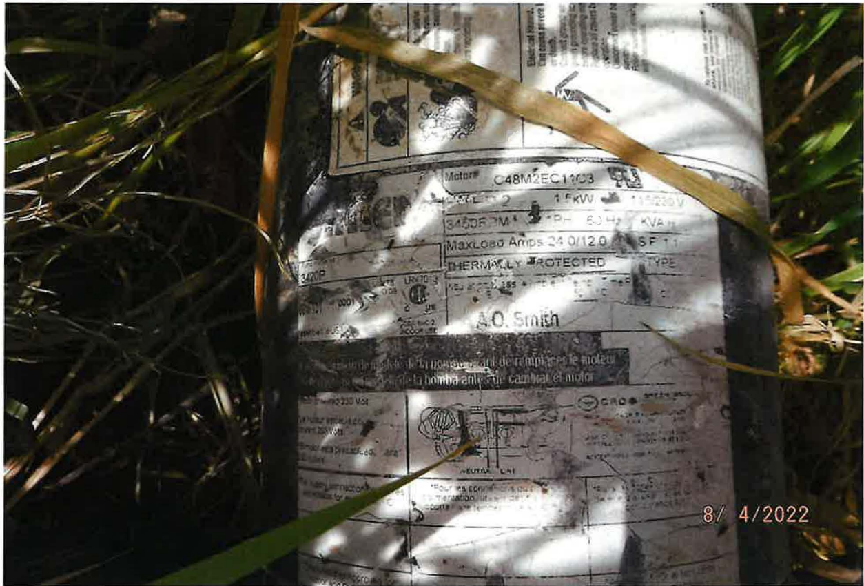
PUMP MOTOR # C48M23C11C3
