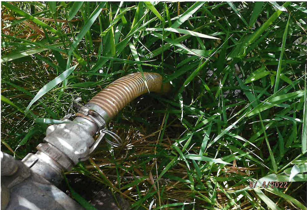
POD – SCREENED INTAKE WITH PUMP FROM S.F. PALOUSE RIVER
