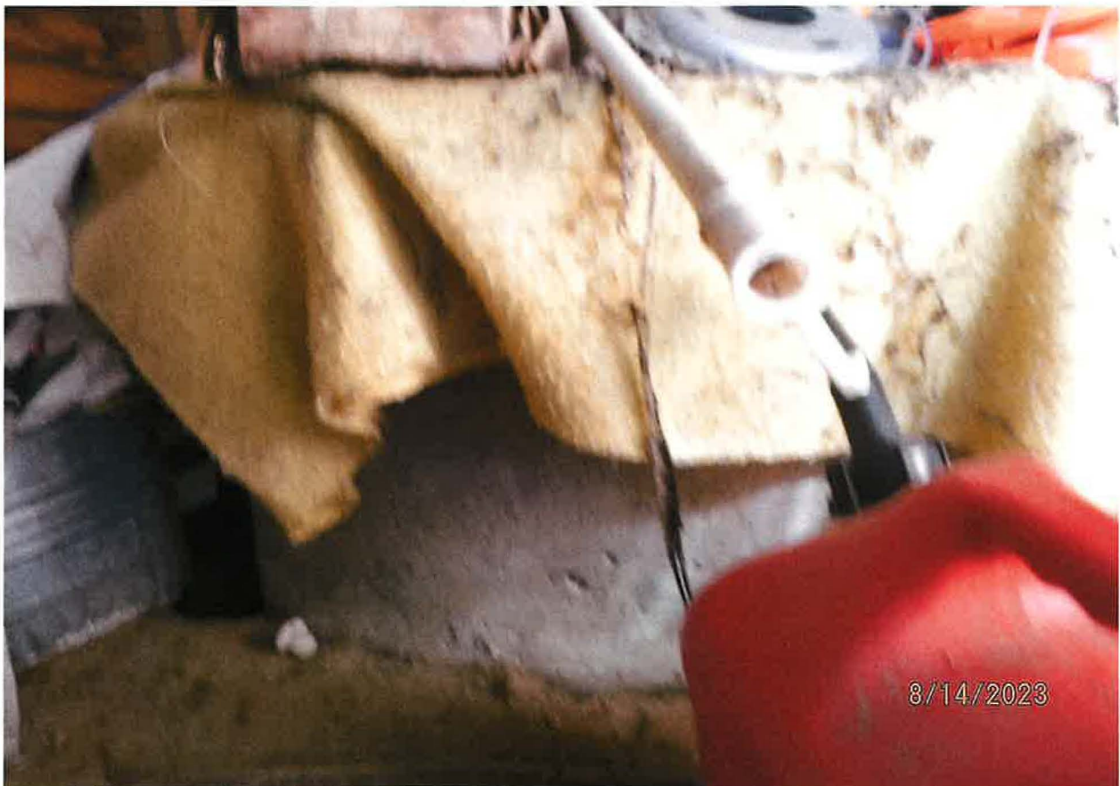
POD – HAND DUG WELL CONSTRUCTED OF CONCRETE RINGS
